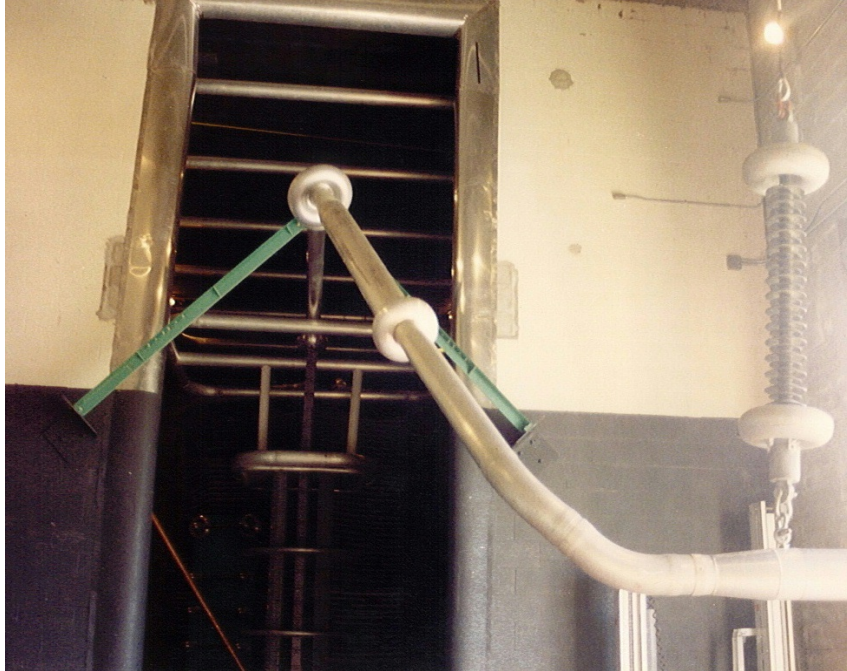
Figure 5-15. Forestport high-voltage feed from helix house.
