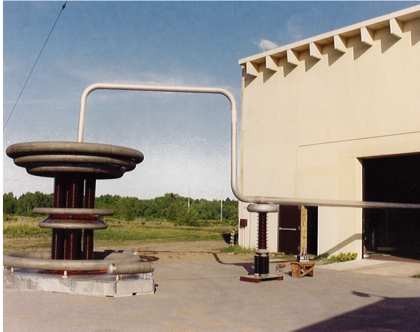
Figure 5-16. Forestport outside test setup.
