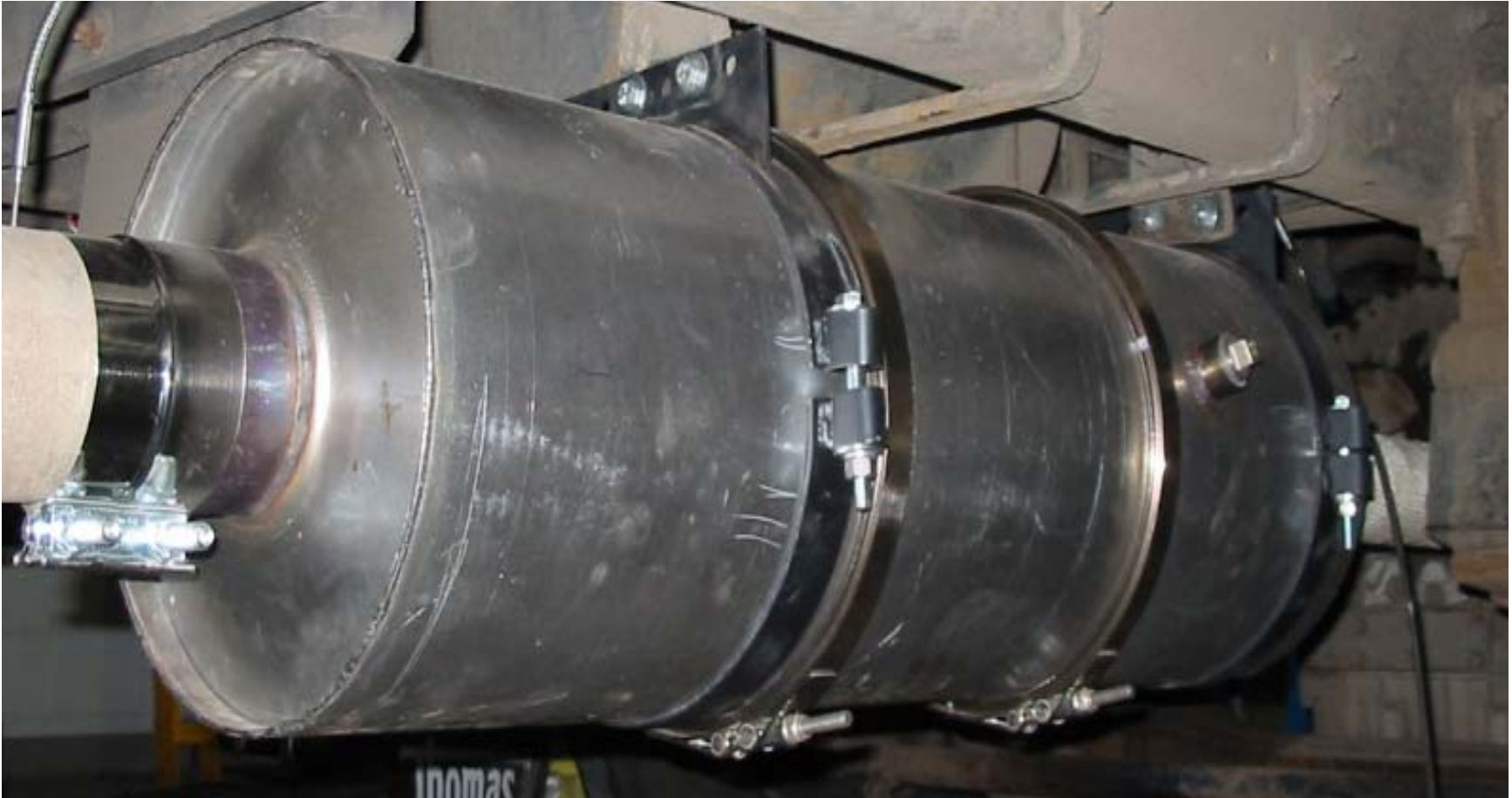
ESW Particulate Reactor Installed
