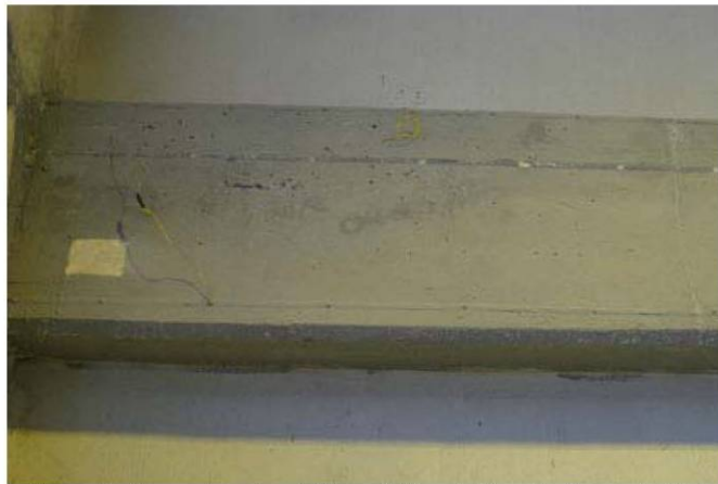
Figure 1h. Closer view of coated beam "A"; note Ti mesh strips, embedded test lead wires, and uncoated rectangular patch
