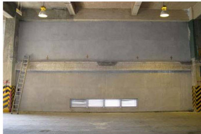
Figure 1f. Overall view of beam "AA" after treatment; reportedly treatment consisted of vapor and liquid inhibitor application to the concrete beam surface
