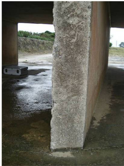
Figure 4. Typical damage on the upstream edges of the culvert #2 piers.
