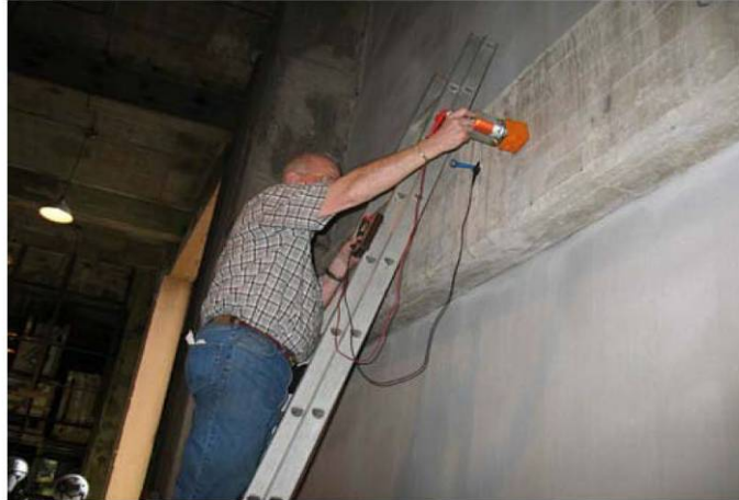
Figure 2b. Measurement of rebar half-cell corrosion potentials on beam "AA" using a copper/copper-sulfate reference electrode before treatment
