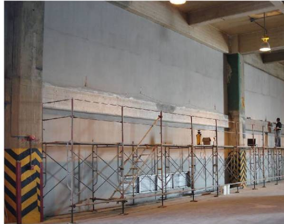
Figure 18. Overview of Beam 1 in July, 2007. Note patch repairs (darker appearance). Compare to Figure 15.
