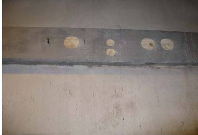
Figure 1i. Closer view of beam "A": showing additional uncoated round patches
