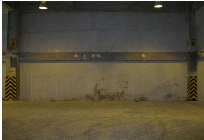
Figure 1g. Overall view of beam "A" after treatment; reportedly a zinc-aluminum-indium rich coating was applied to the concrete beam surface
