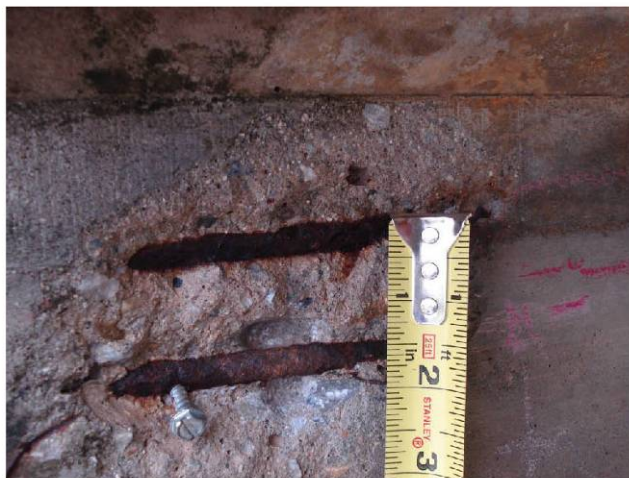
Figure 2. Exposed rebar on Culvert #2.
