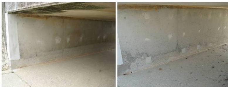
Figure 14. Typical appearance of culvert before (left) and 6 months after (right) inhibitor application.
