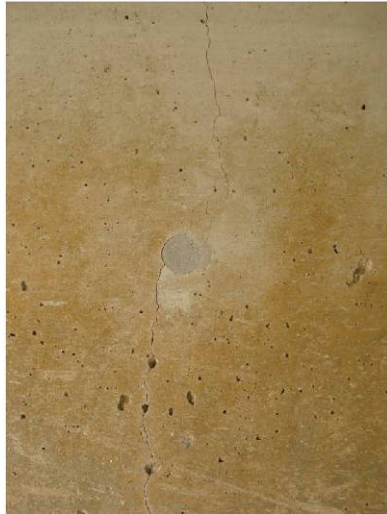
Figure 3. Typical pier wall surface containing a crack and plugged area.
