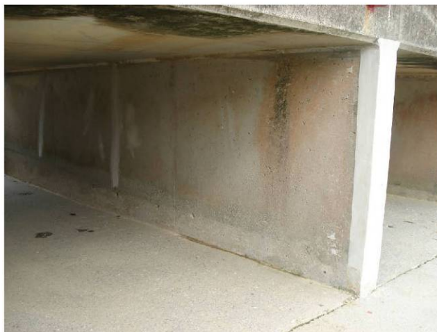
Figure 12. Typical previously repaired areas (lighter mortar) on Culvert #3.
