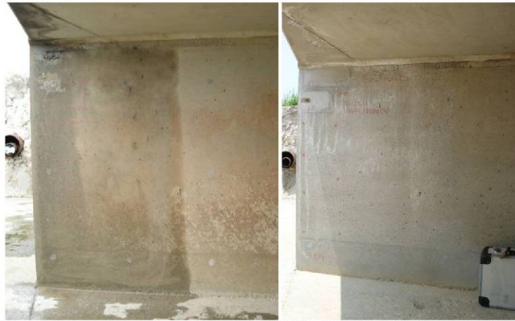
Figure 5. Typical appearance of culvert before (left) and 6 months after (right) inhibitor application.
