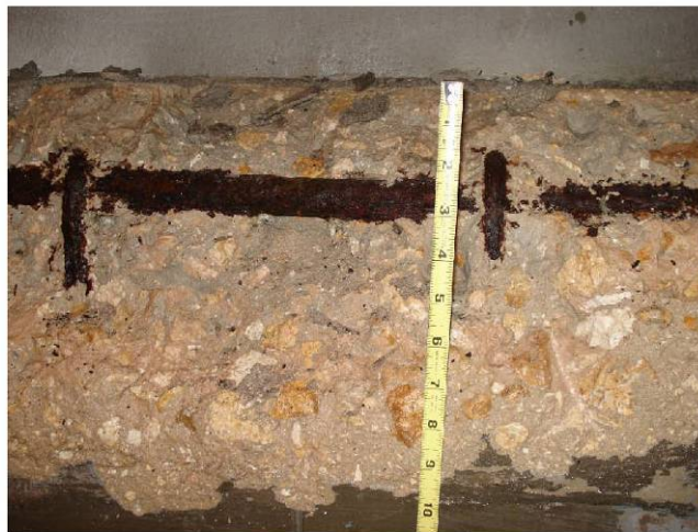
Figure 17. Representative exposed rebar at a repair location.
