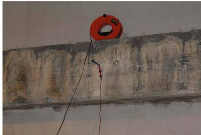
Figure 2a. Photo showing steel awl connection to rebar in beam "A" before treatment
