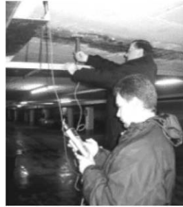
GalvaPulse corrosion rate measurement at a leaking joint
