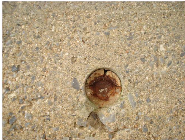
Figure 13. Typical steel within a delaminated "plug."
