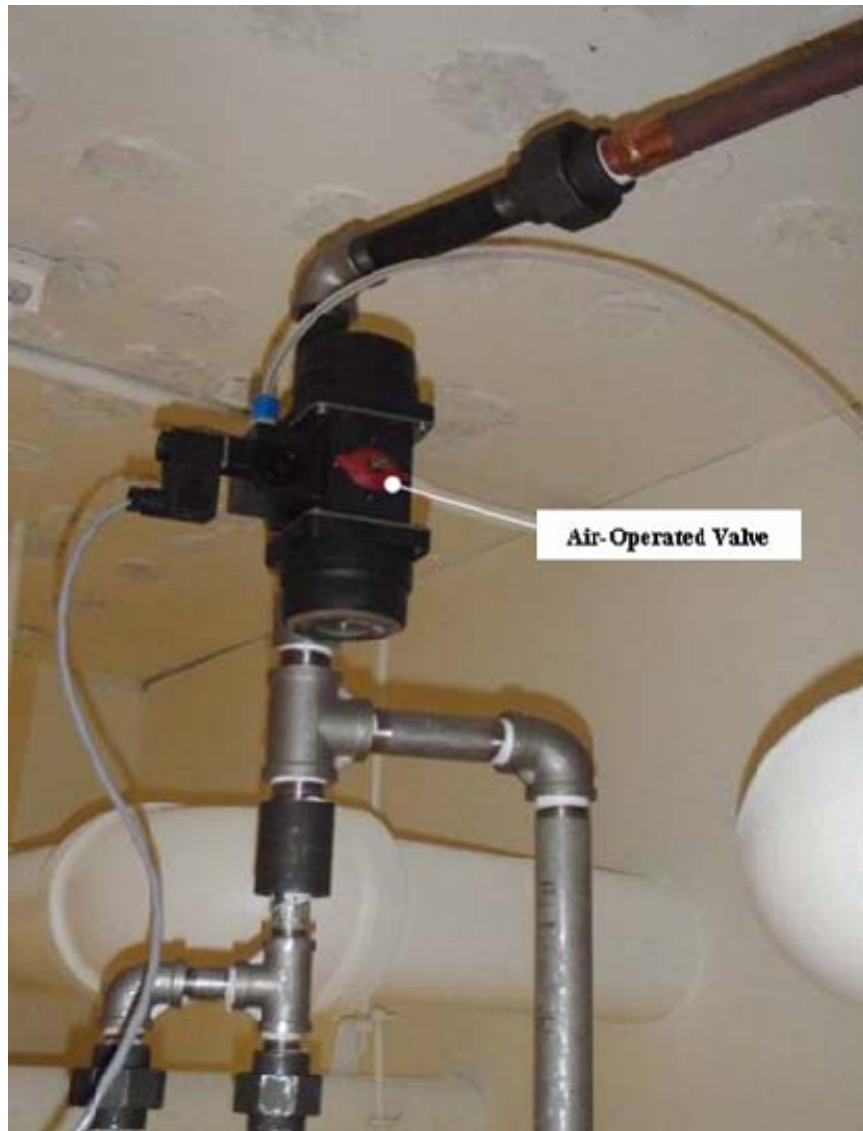
Figure 14. Exhaust System's Pneumatic Ball Valve
