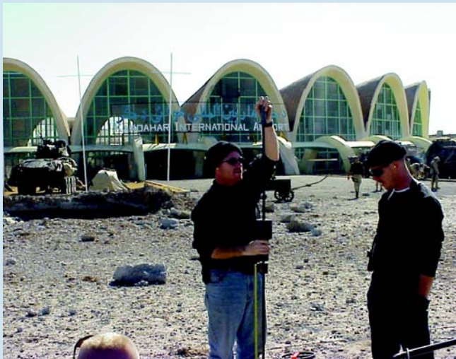
TSgt Steven Russell and TSgt Greg Crosslin conduct pavement tests using a dynamic cone penetrometer at Kandahar International Airport, Afghanistan.
