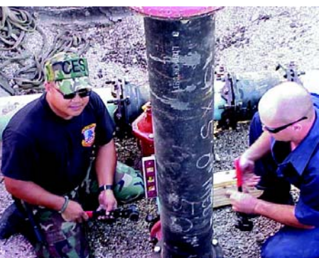
(From top to bottom) The pit of well number 1 on Aug 4, 2001. This is where Randolph's water contamination problems began. (Photo by A.C. Thomas) SrA Shaun Ballor, 37th CES equipment operator, stands by as emergency repairs are made to Randolph's water lines. (Photo by CMSgt Kenneth Thomas) TSgt Duane Cruz (left), 12th CES, and TSgt David Riggs, 37th CES, repair a section of broken pipe. (Photo by CMSgt Ercilia Ramos)
