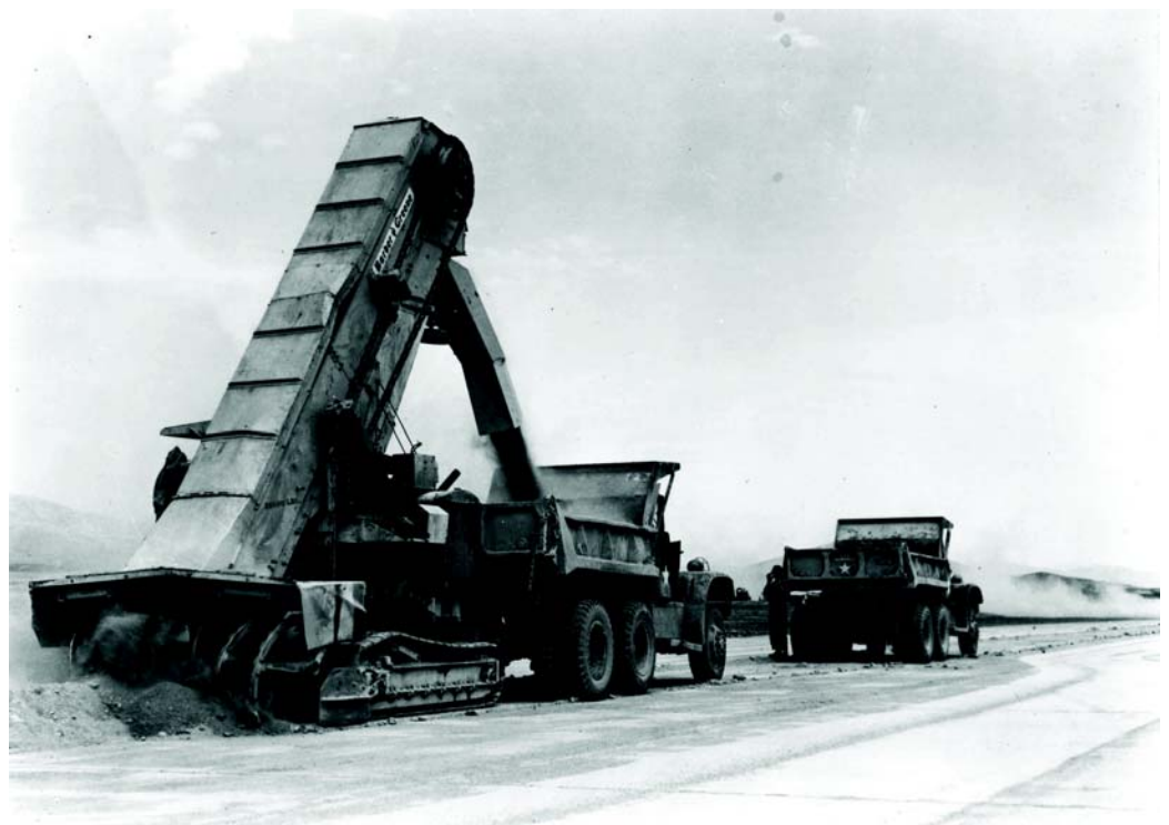
Trucks use a self-propelled conveyor loader to remove the curing sand from a 9,000-foot runway completed by the 930th EAG. (USAF photo)
