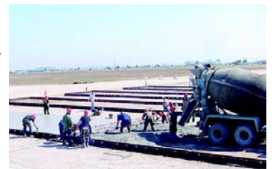
Craftsmen pour alternating concrete pad sections for Kunsan's hazardous cargo marshalling pad. The 554th completed the $475,000 project in 2001.
