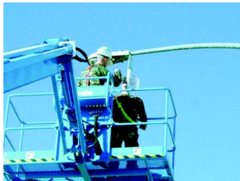
The 50th CES heads an aggressive MILCON program resulting in the largest amount of infrastructure growth Schriever AFB has seen since its inception in 1985.
