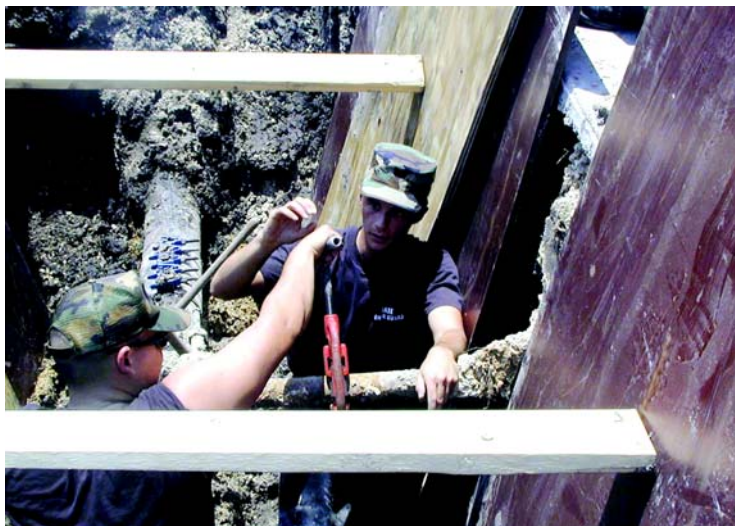
MSgt Luis A. Adams is the non-commissioned officer in charge of infrastructure for the 12th CES, Randolph AFB, TX.
