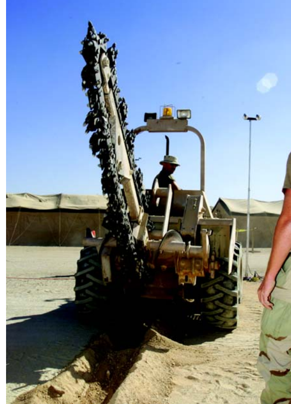
Digging a trench at a forward-deployed location Nov. 9. (Photo by TSgt Marlin Zimmerman)
