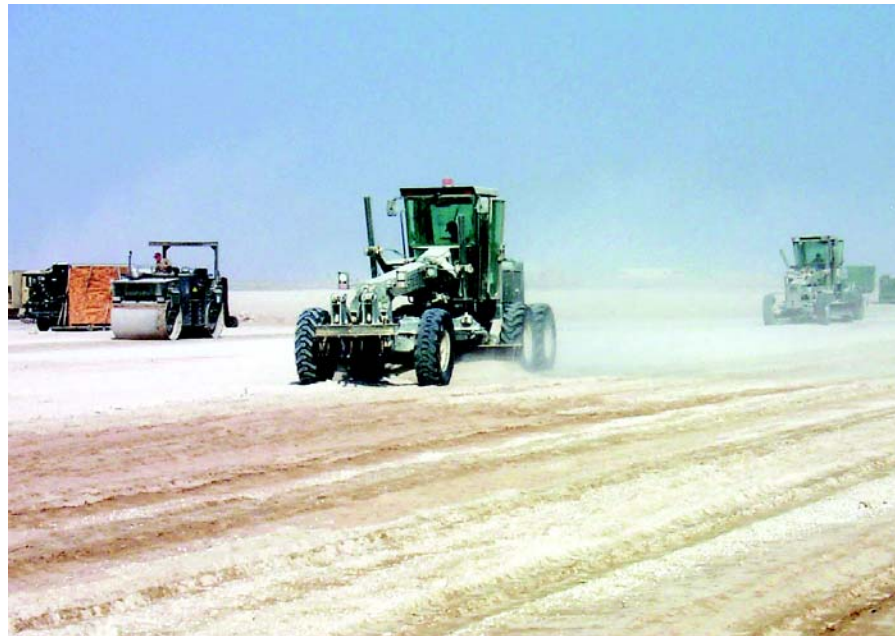
(From left) SSgts Tracy McBride and Jeramy Isaac and A1C Ryan O’Connell, all from the 823rd RHS, construct an equipment marshalling area for the air terminal operations center at a deployed location. (Photo by TSgt Carole Steele)
