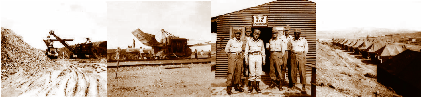
Snapshots provided by 1st Lt Fred Williamson (second from left in third picture) show the 839th EAB using power shovels to load gravel and rock into dump trucks for transporting to the rock crusher; loading crushed rock into a concrete mixer; officers of C Company, 839th EAB, in front of the company orderly room; and one of the rudimentary army camps where aviation engineers lived. Camps were composed of squad-sized tents for enlisted personnel and metal buildings for company orderly rooms, battalion and group headquarters, mess halls and armories.
