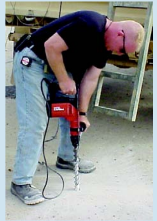
TSgt Jody Root uses a Hilti drill to determine the thickness of the airfield pavement at Kandahar International Airport, Afghanistan. (Photos courtesy Airfield Pavements Evaluation Team)
