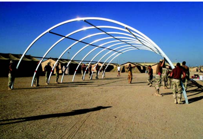
Deployed 552nd CES members erect a California tent during Operation ENDURING FREEDOM, Oct. 30. (Photo by A1C Maryann Walker)
