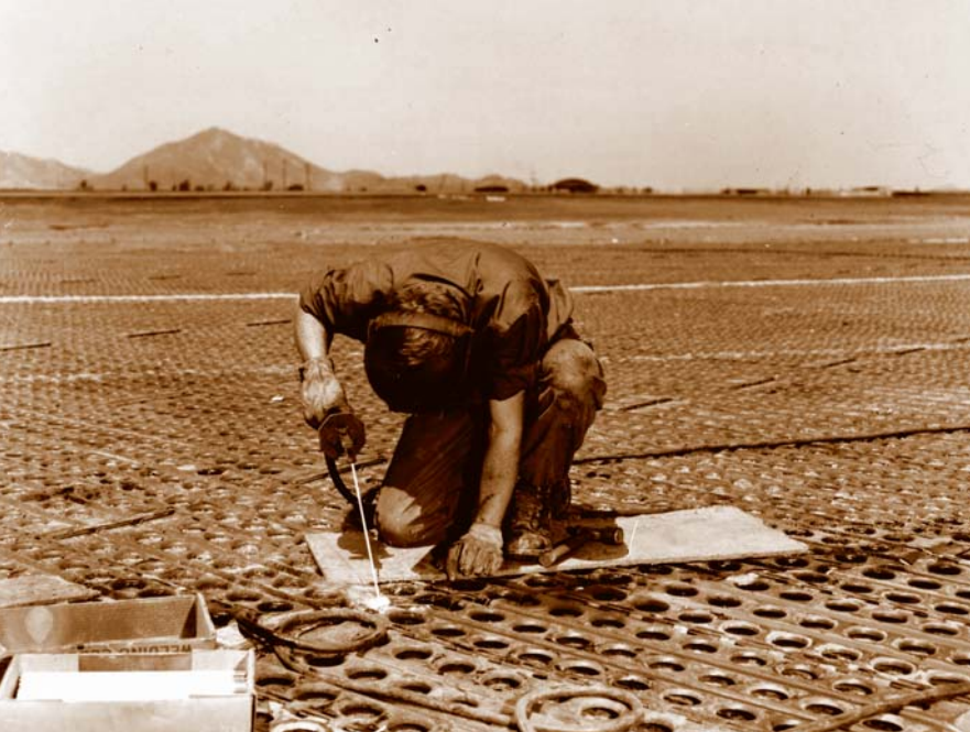
Repair and maintenance of pierced steel planking was a constant job on Korean airfields that saw up to 10,000 takeoffs and landings per month. (All photos USAF unless otherwise noted)
