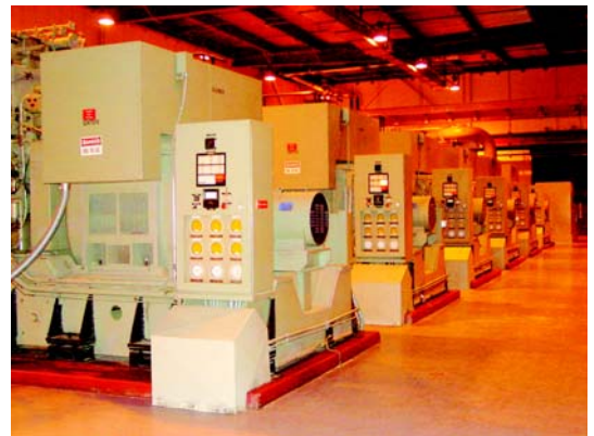
A total of seven diesel generators make up Schriever’s power plant and produce an astounding 15 megawatts of power.
