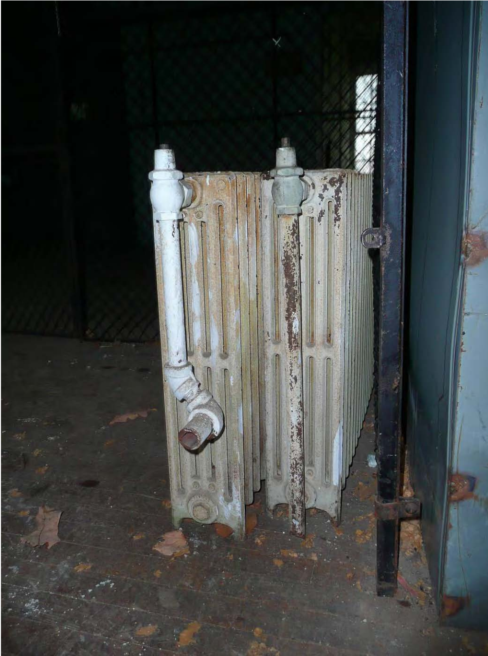
Photo 42 – example of radiator on first floor
