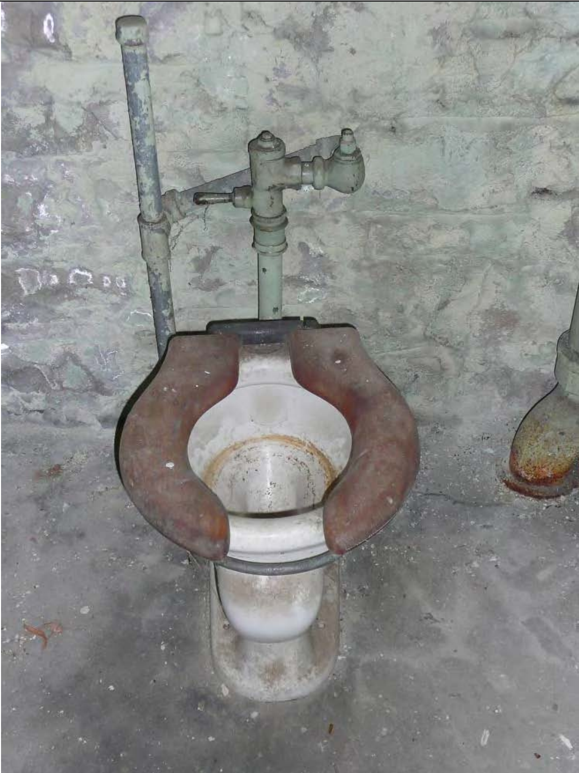
Photo 30 – toilet in second floor bathroom
