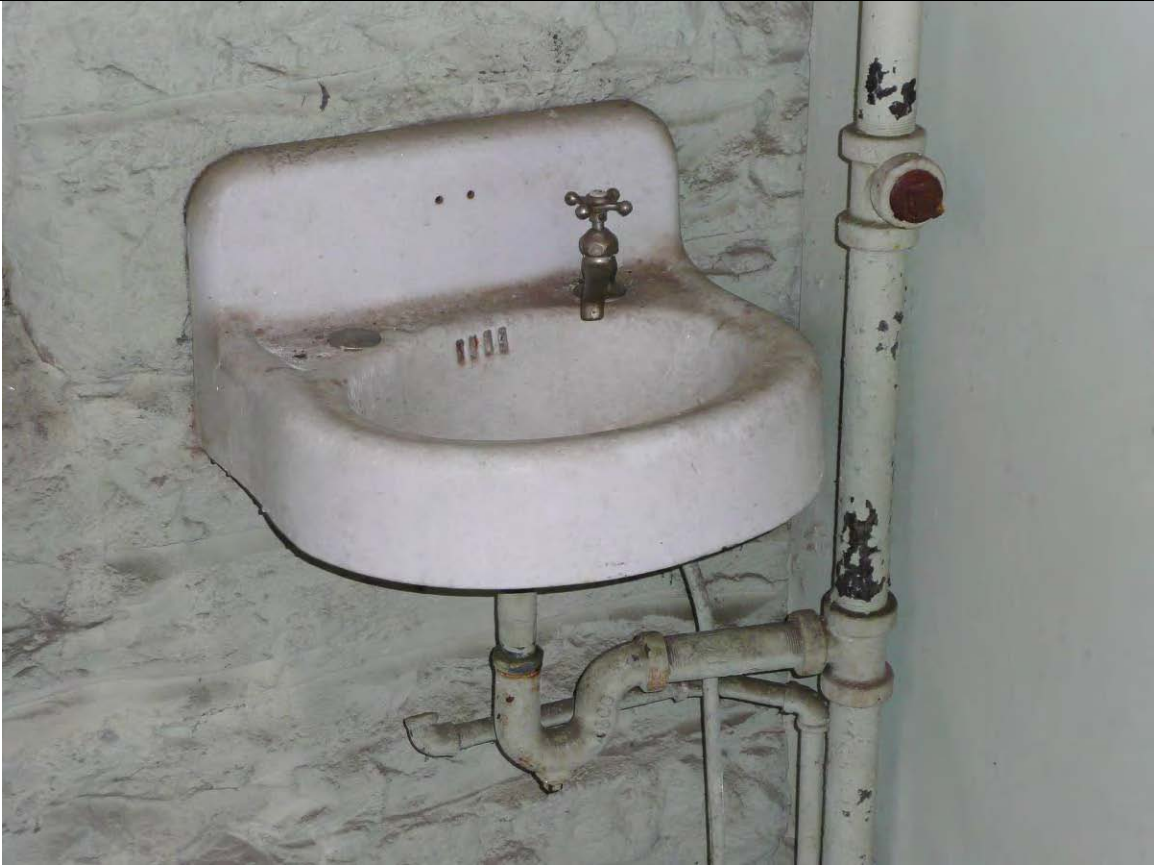
Photo 32 – sink in second floor bathroom
