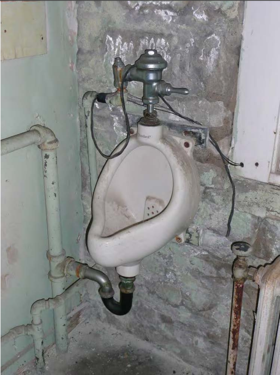
Photo 31 – urinal in second floor bathroom
