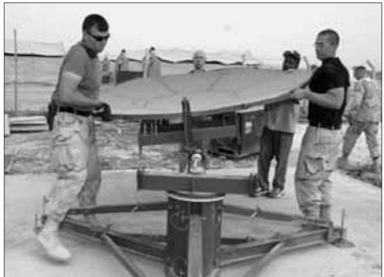
Members of the 407 Expeditionary Communications Squadron put together a Flyaway KU Band Earth Terminal (FKET) Satellite System. The 407 ECS is deployed to Tallil Air Base, Iraq. U.S. Air Force photo by Airman 1st Class Desiree N. Palacios.
