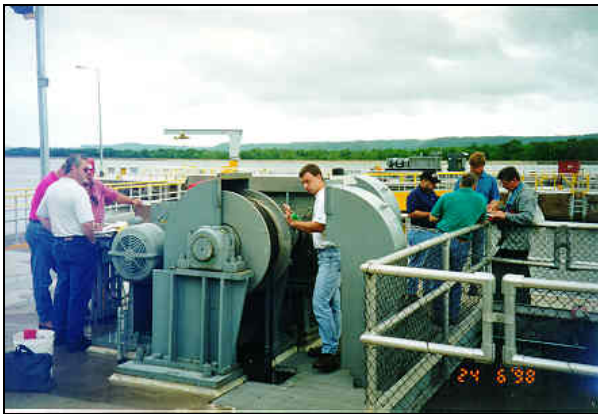
Illustration 12. Lock and dam operating equipment.
