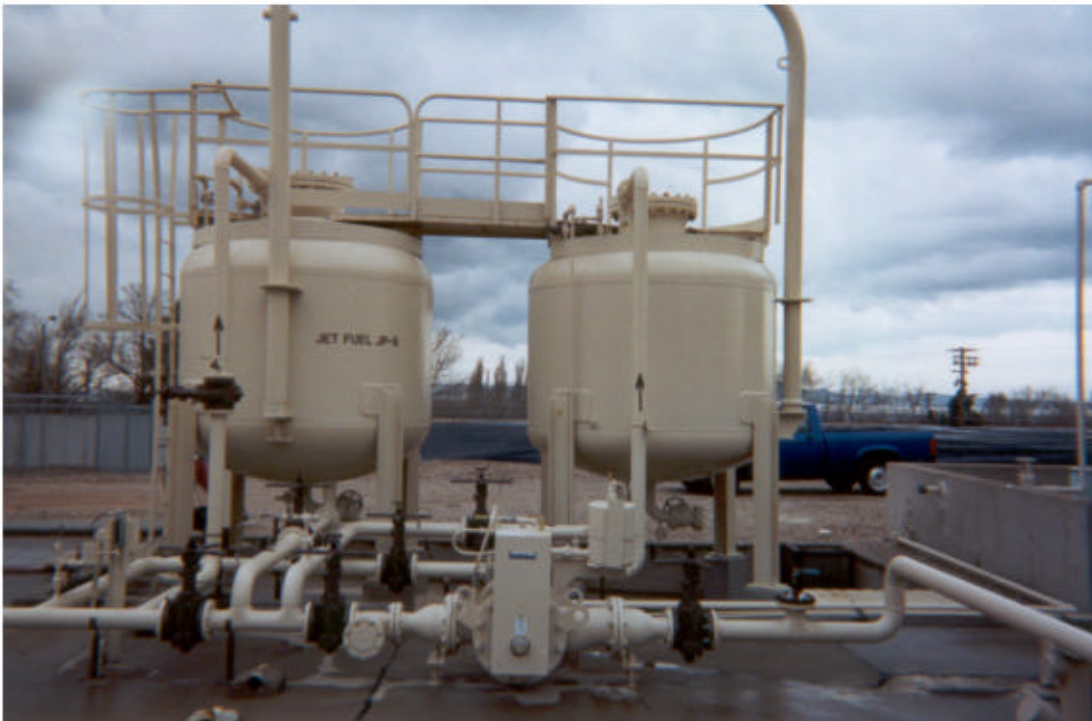
Figure 4. Clay Filters at Hill AFB
