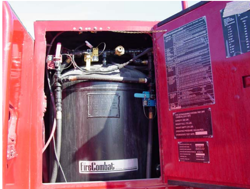
Figure 3.6.1: The 500 lb dry chemical storage tank located behind the passenger's side cab.
