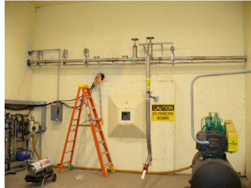
Figure 8: LH2 supply line
