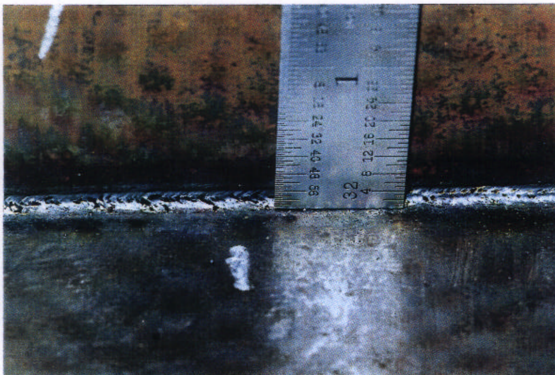
25. Close-up of autogenous weld
