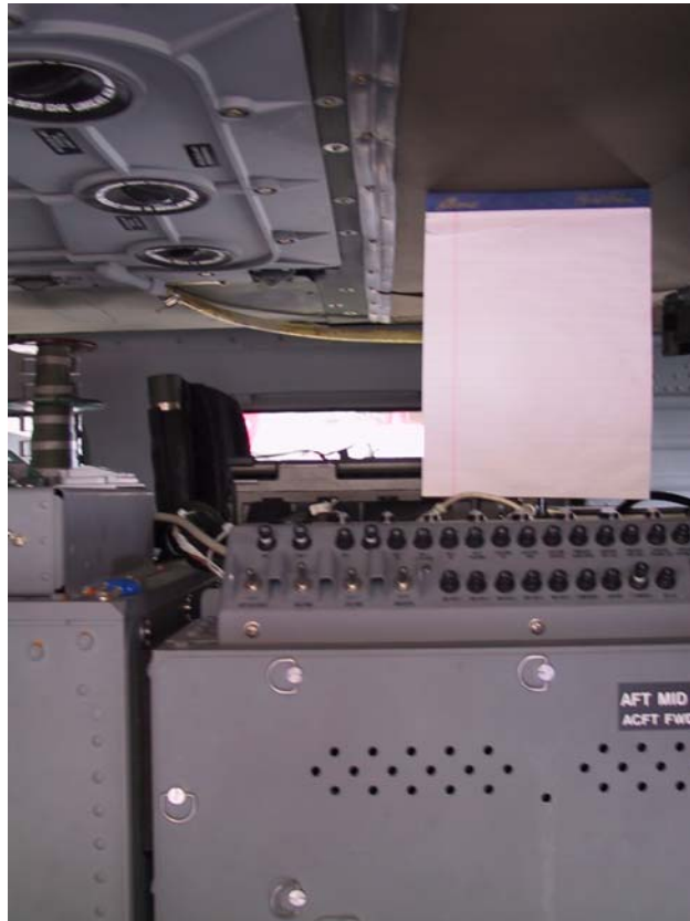
Figure 23. Restricted space above center rack.
