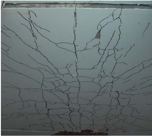
Figure 16. Internal damage from Round 2
