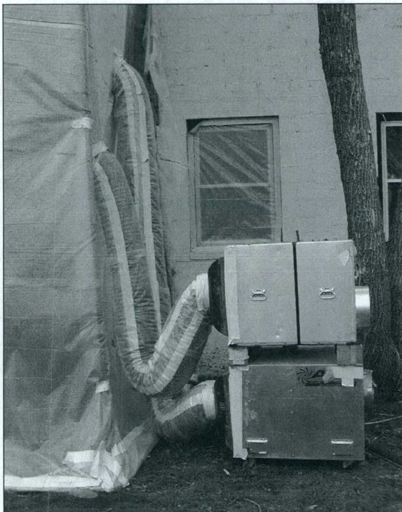
Figure 3. Ventilation units and ducts attached to end of containment.
