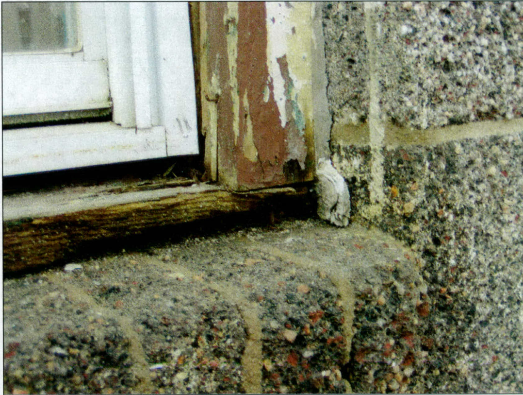
Figure 9. Incidental damage to wood window frame caused by wet abrasive blasting.
