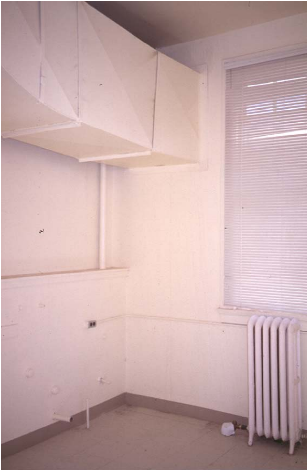
Photograph 50. Building 7157 cooling equipment.
