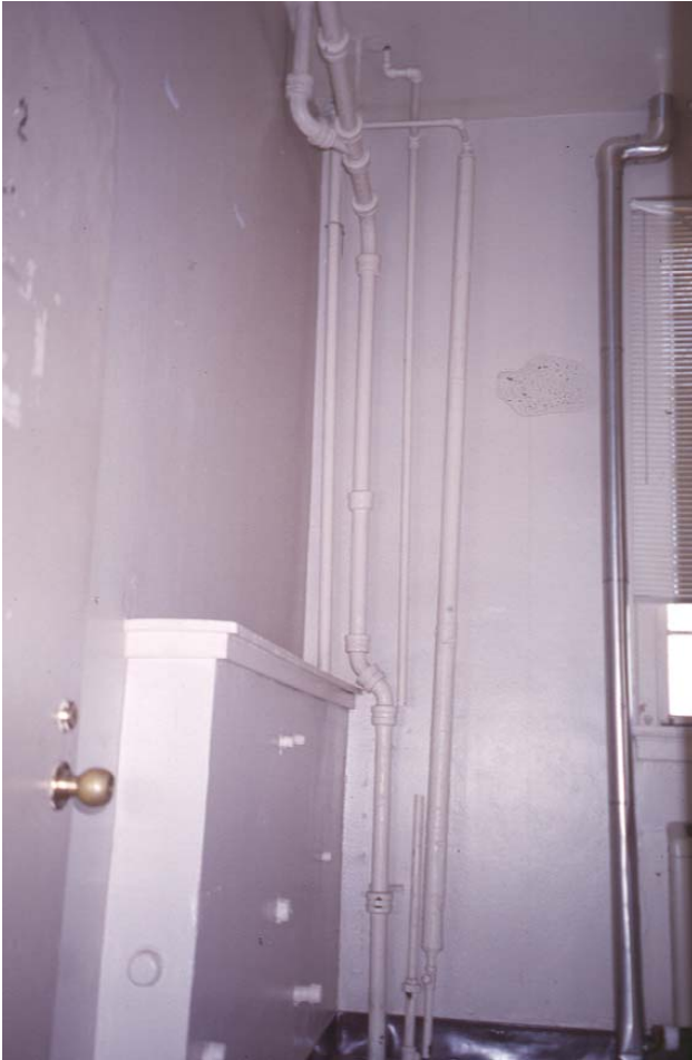
Photograph 49. Non-historic plumbing modifications in Building 7157.
