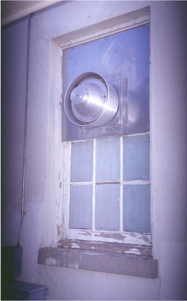
Photograph 43. Non-historic washroom window modification.
