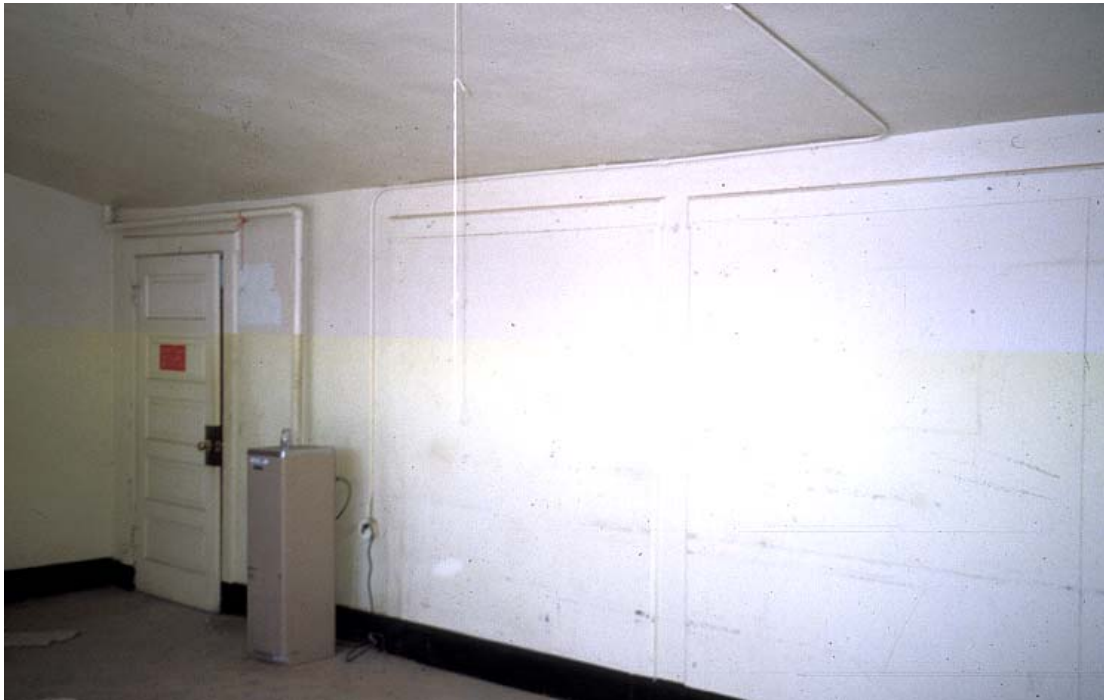
Photograph 30. Historically incompatible modifications of gymnasium locker room portal.
