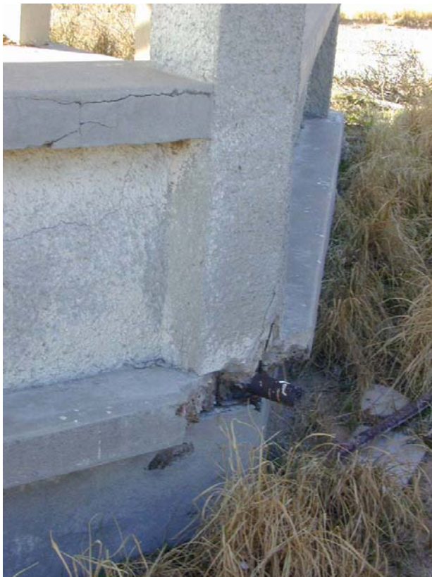
Photograph 3. Detail of exposed concrete reinforcement on bandstand.
