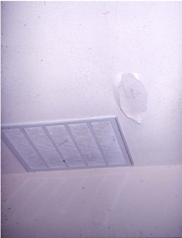
Photograph 66. Water stain on BOQ ceiling.
