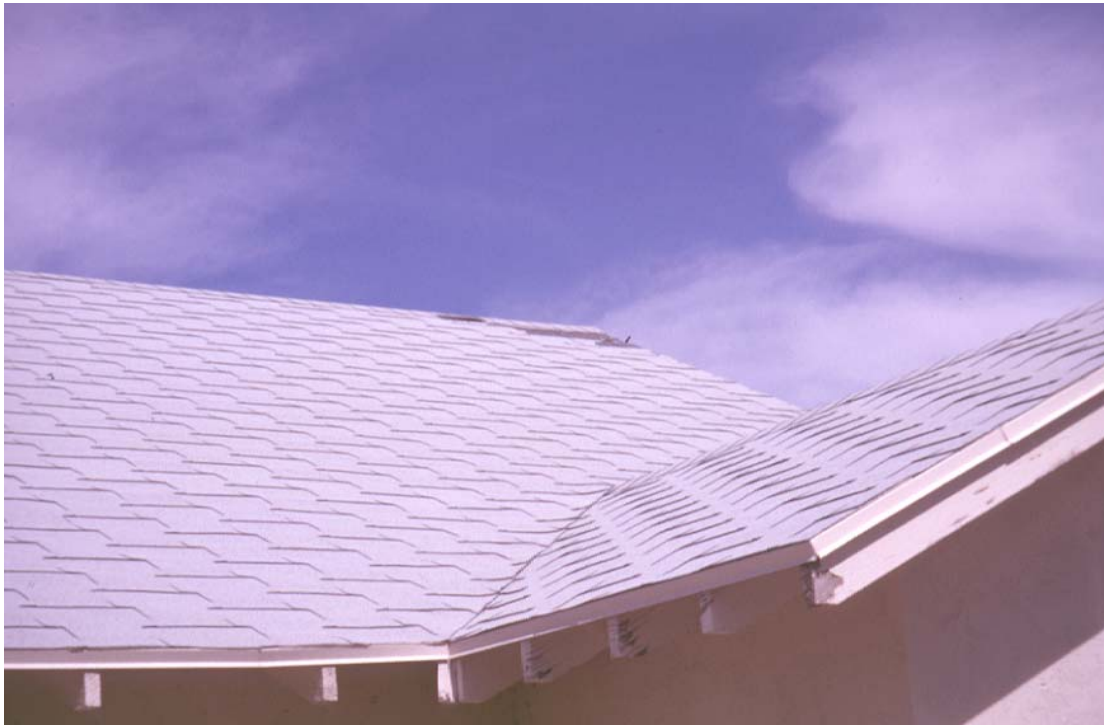
Photograph 65. Shingles missing on BOQ roof ridge.
