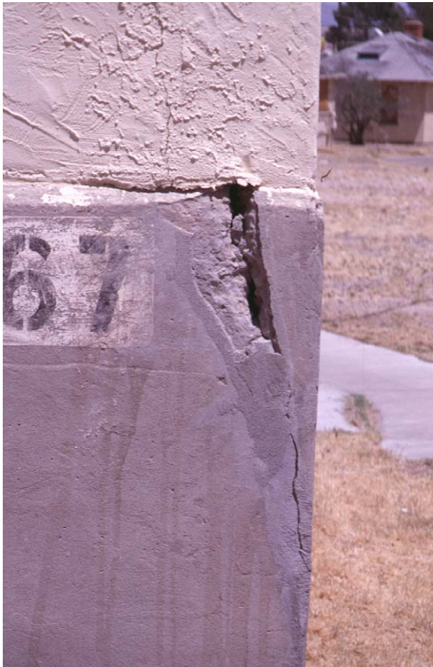
Photograph 71. Conference center foundation crack.
