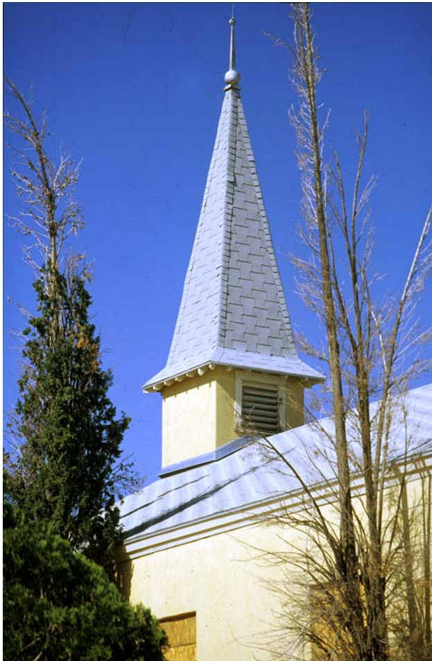
Photograph 7. Minor stucco cracking on chapel.
