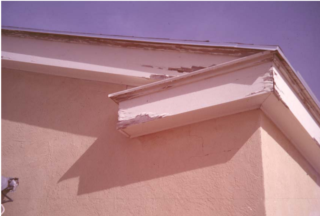
Photograph 17. Deterioration of theater eave trim.
