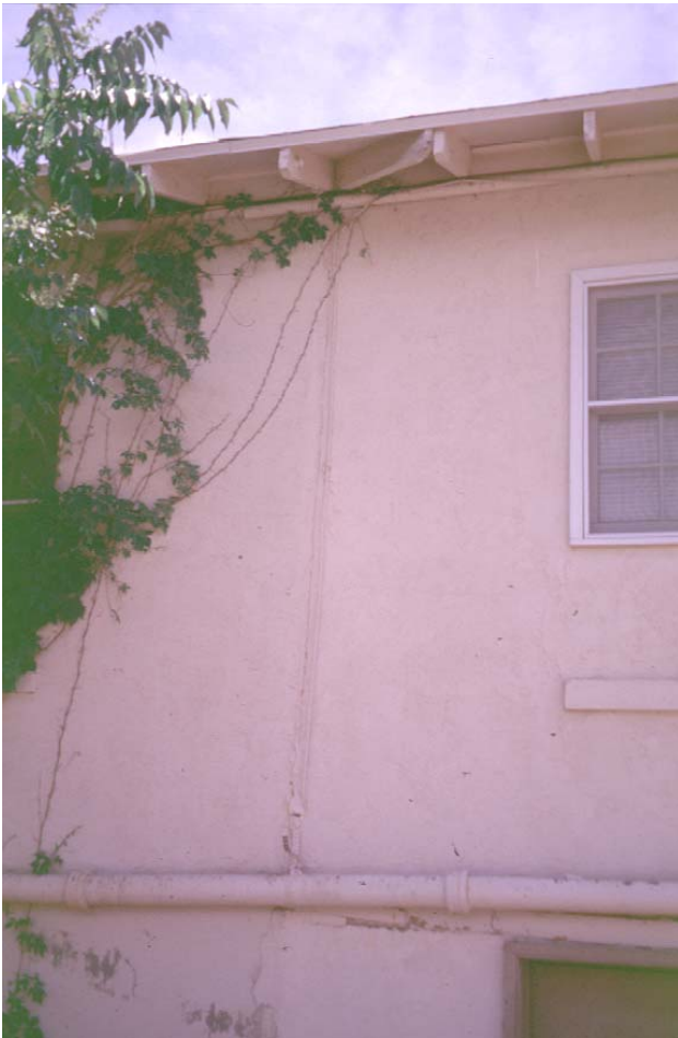
Photograph 62. Minor BOQ wall crack.
