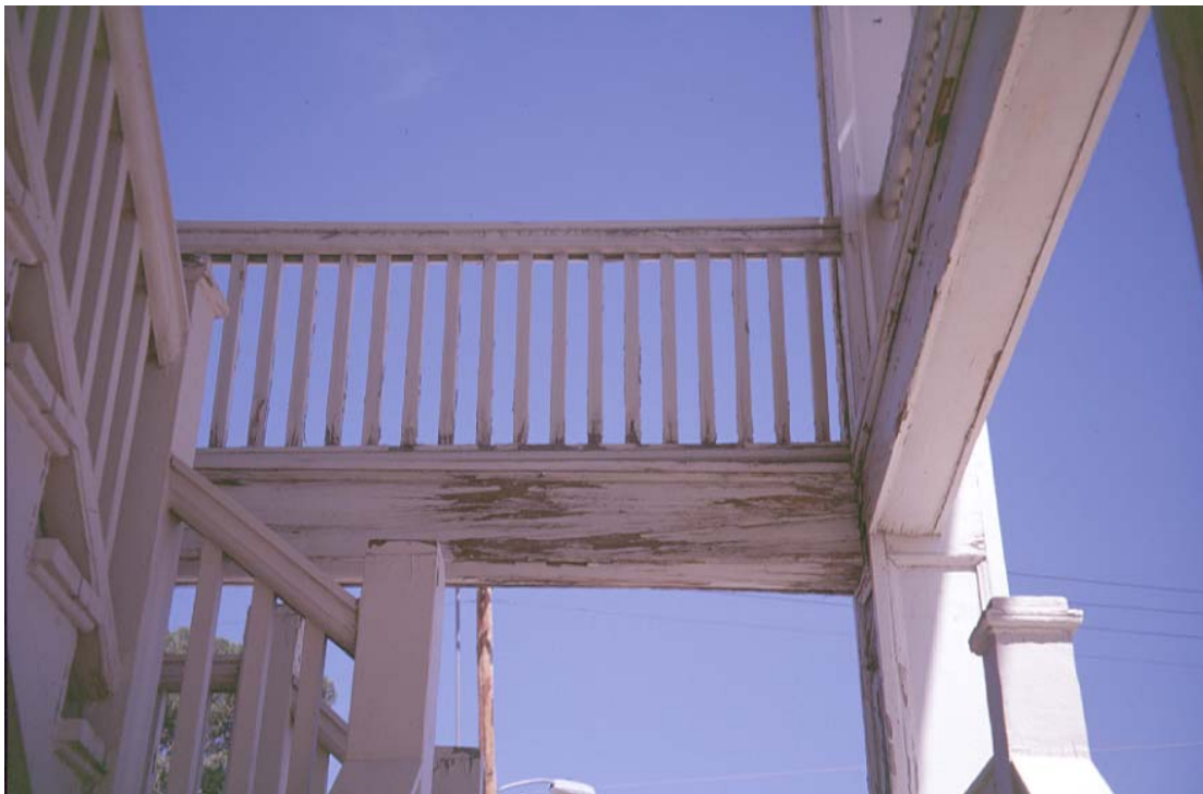
Photograph 40. Typical deteriorated exterior trim on barracks.
