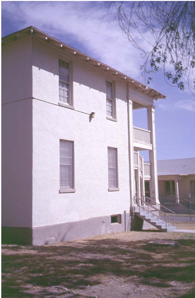
Photograph 58. Non-historic modification of Building 7159 exterior stairways.
