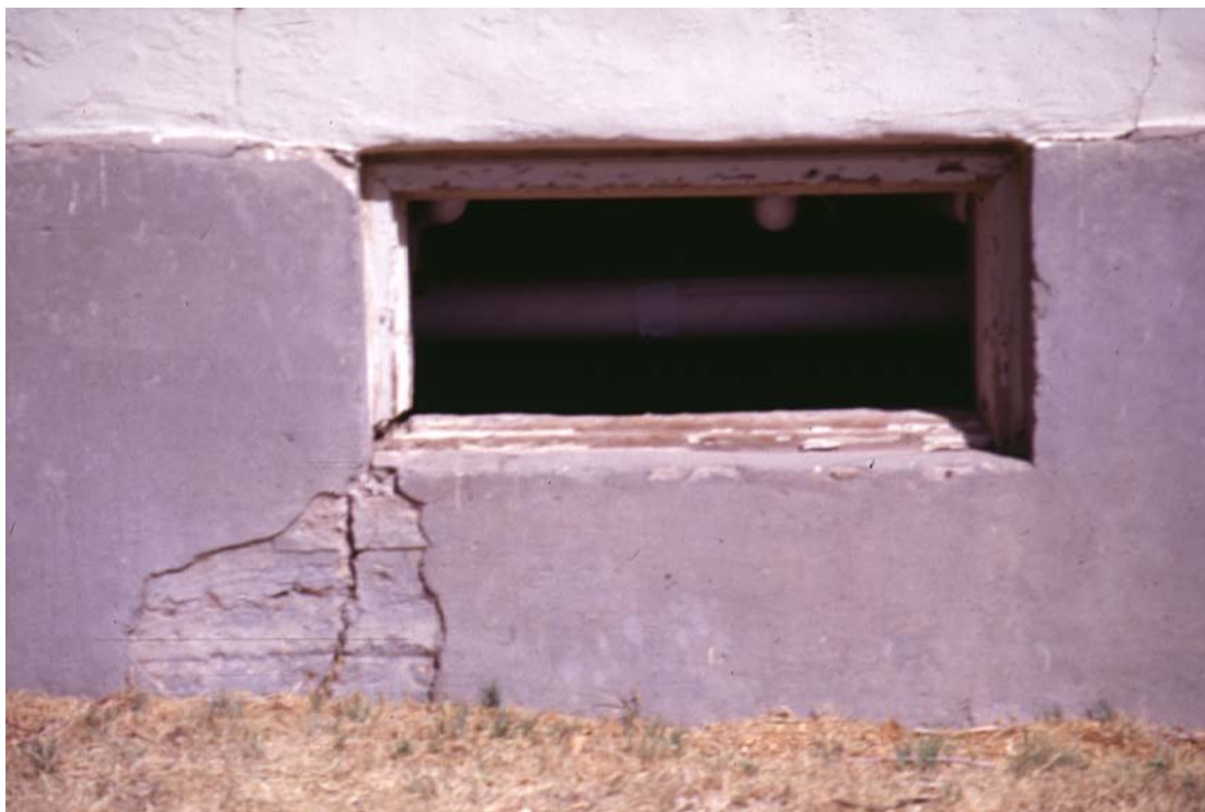
Photograph 54. Building 7159 foundation crack.
