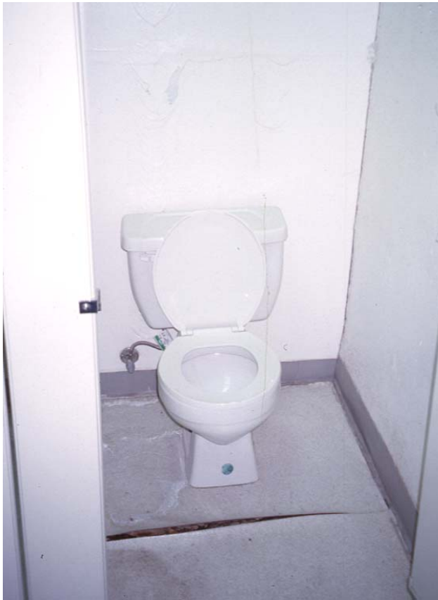
Photograph 53. Damaged vinyl flooring in Building 7158 washrooms.
