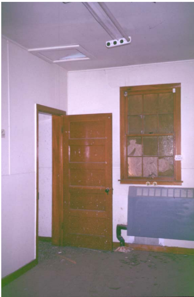
Photograph 8. Damaged sacristy window sashes.
