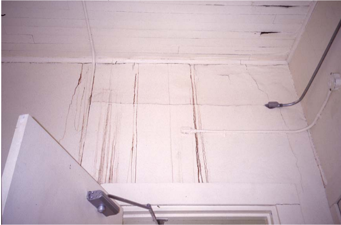
Photograph 48. Signs of roof leakage in porch of Building 7157.
