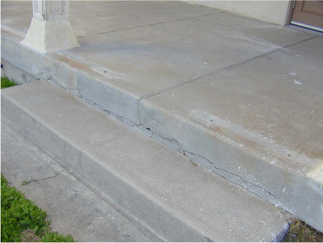
Photograph 72. Crack in north porch slab of Conference Center.
