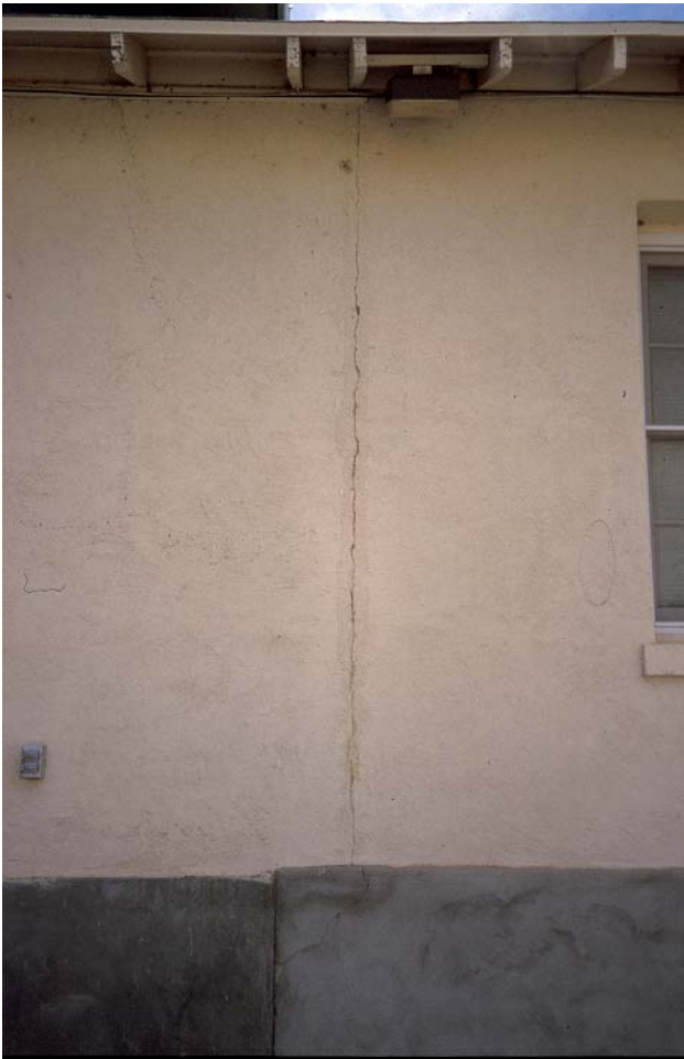
Photograph 61. BOQ foundation and wall crack.
