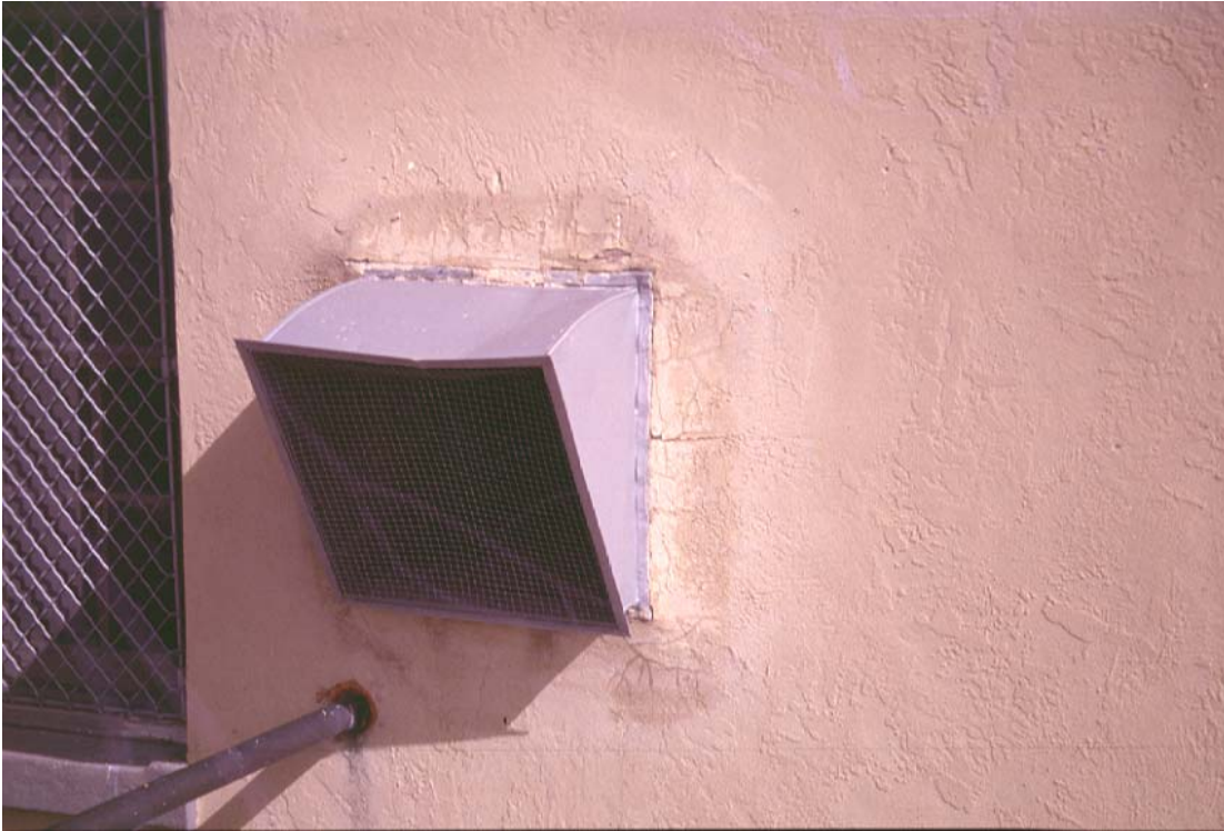
Photograph 16. Minor theater wall cracking around vent hood.
