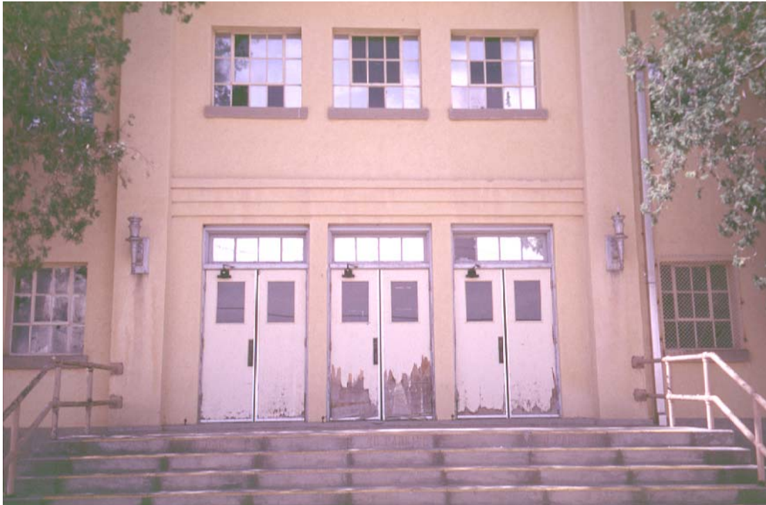
Photograph 26. Deteriorated gymnasium entry doors.
