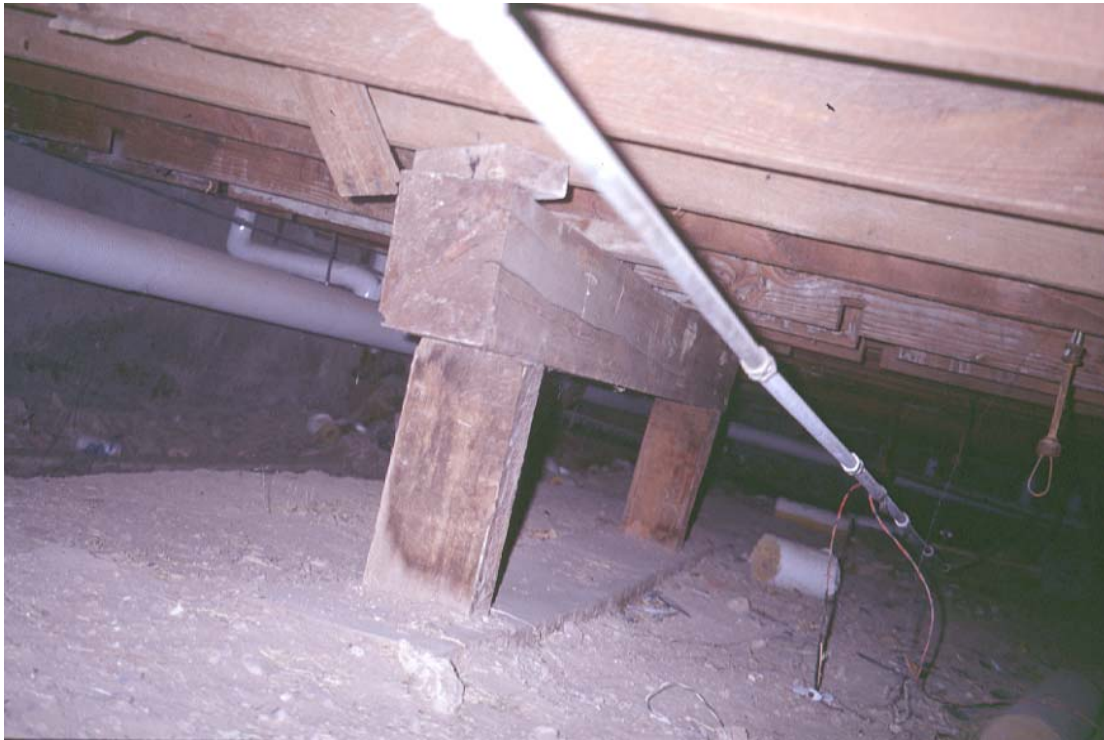
Photograph 56. Makeshift repair of floor framing under Building 7159.
