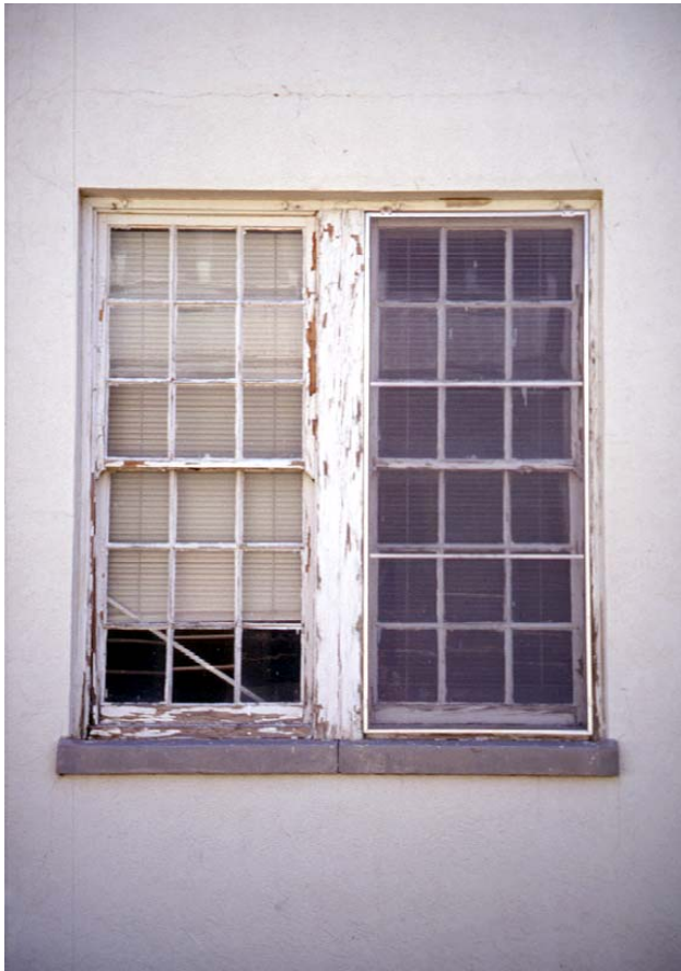
Photograph 42. Seriously deteriorated barracks windows.
