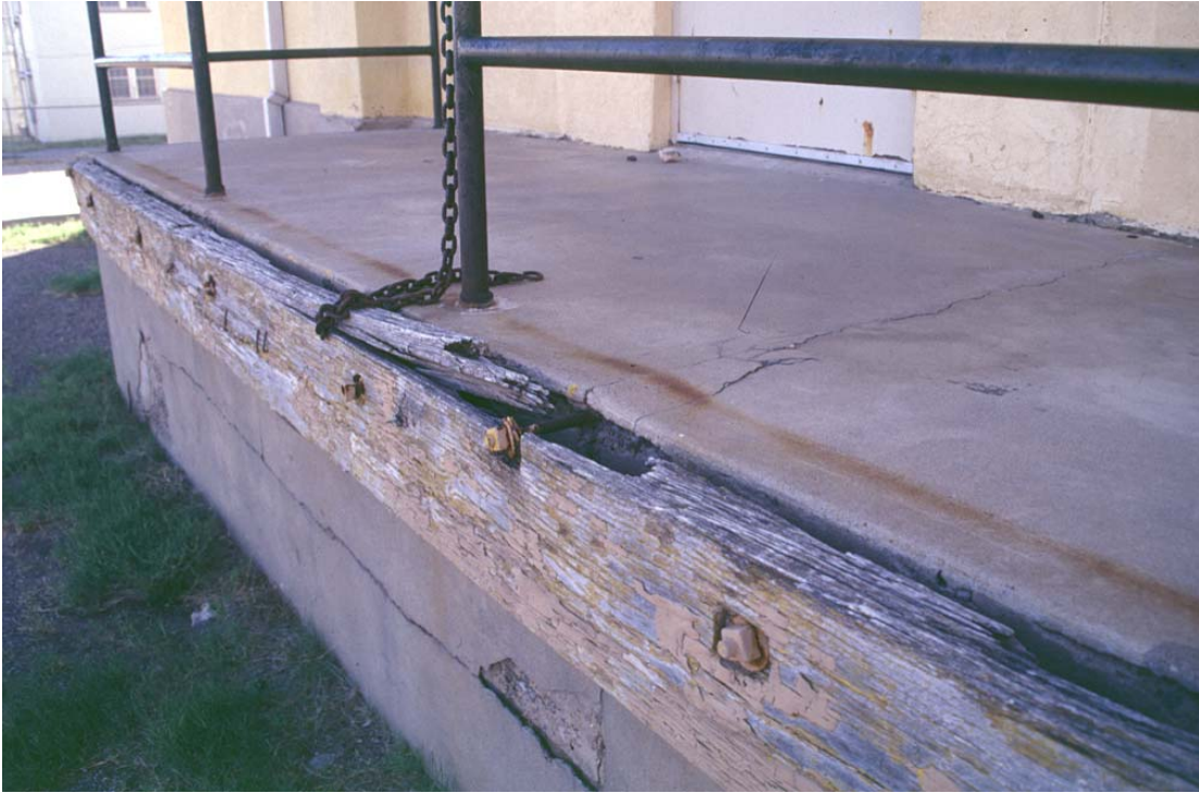
Photograph 22. Concrete damage on gymnasium loading dock.
