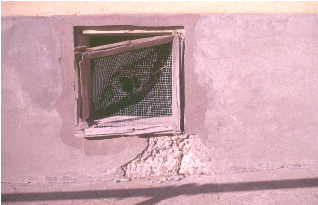
Photograph 20. Minor gymnasium foundation cracking.
