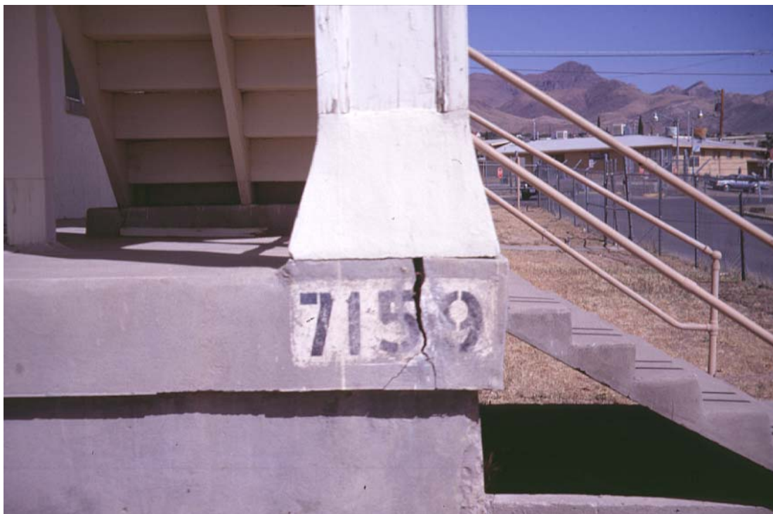
Photograph 34. Detail of barracks porch slab cracks.
