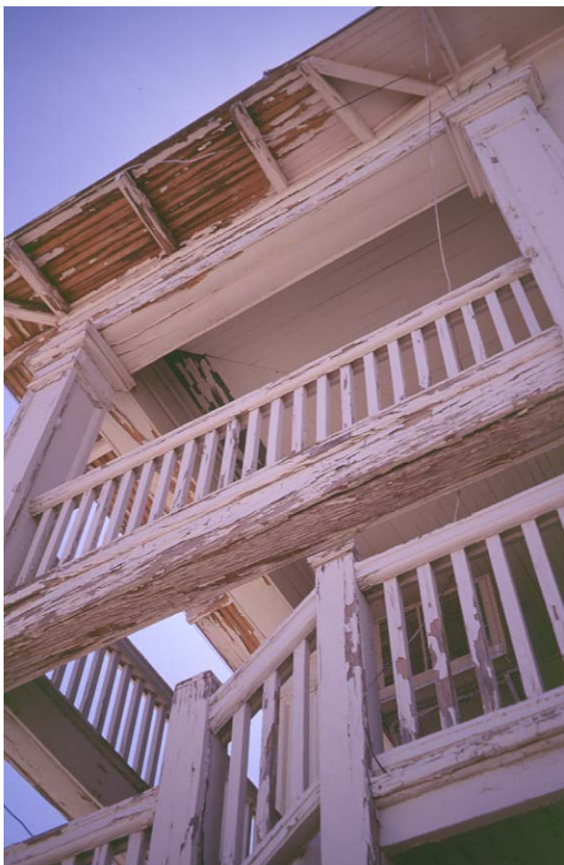
Photograph 38. Typical water damage to barracks porch roof.
