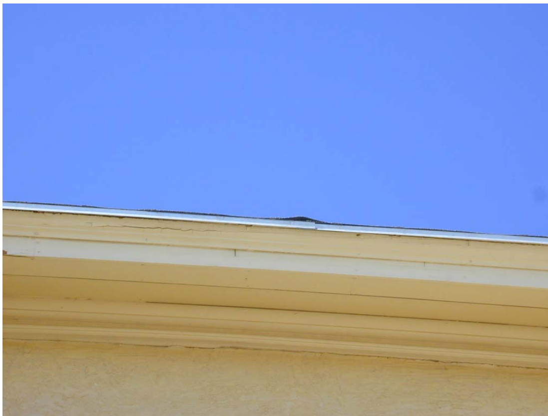
Photograph 28. 'Fish-mouth' shingle warpage on gymnasium gable.
