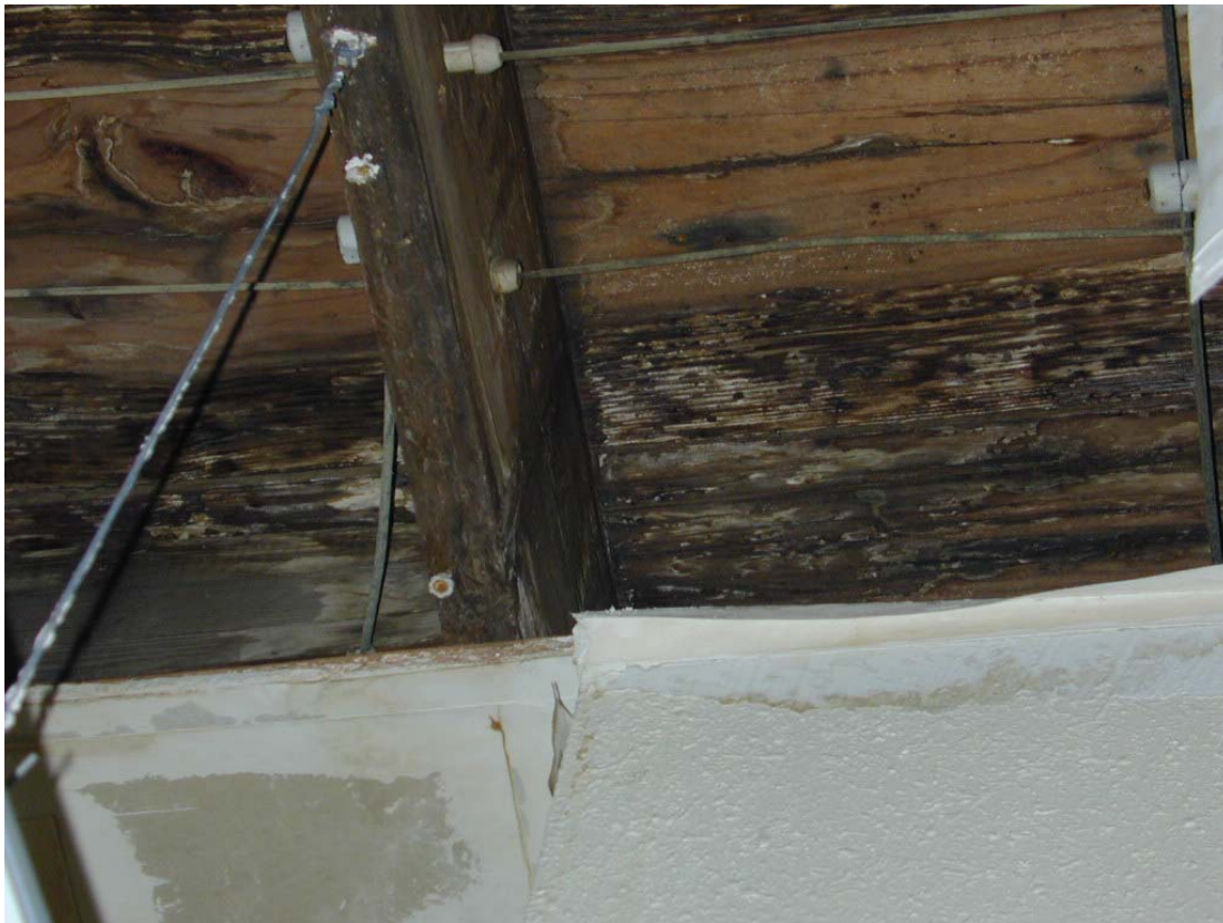
Photograph 35. Water damage from leaking barracks washroom fixtures.
