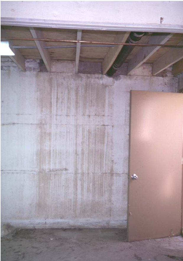
Photograph 69. Water damage on BOQ basement wall from runoff.
