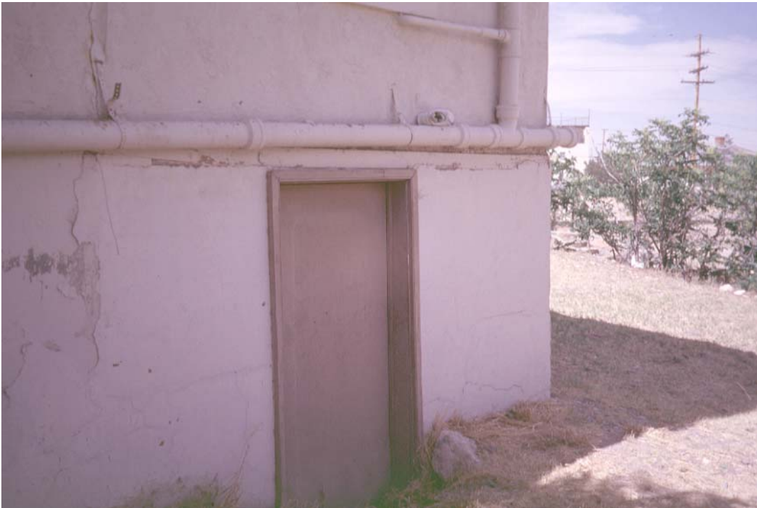
Photograph 64. Deteriorated BOQ basement door.
