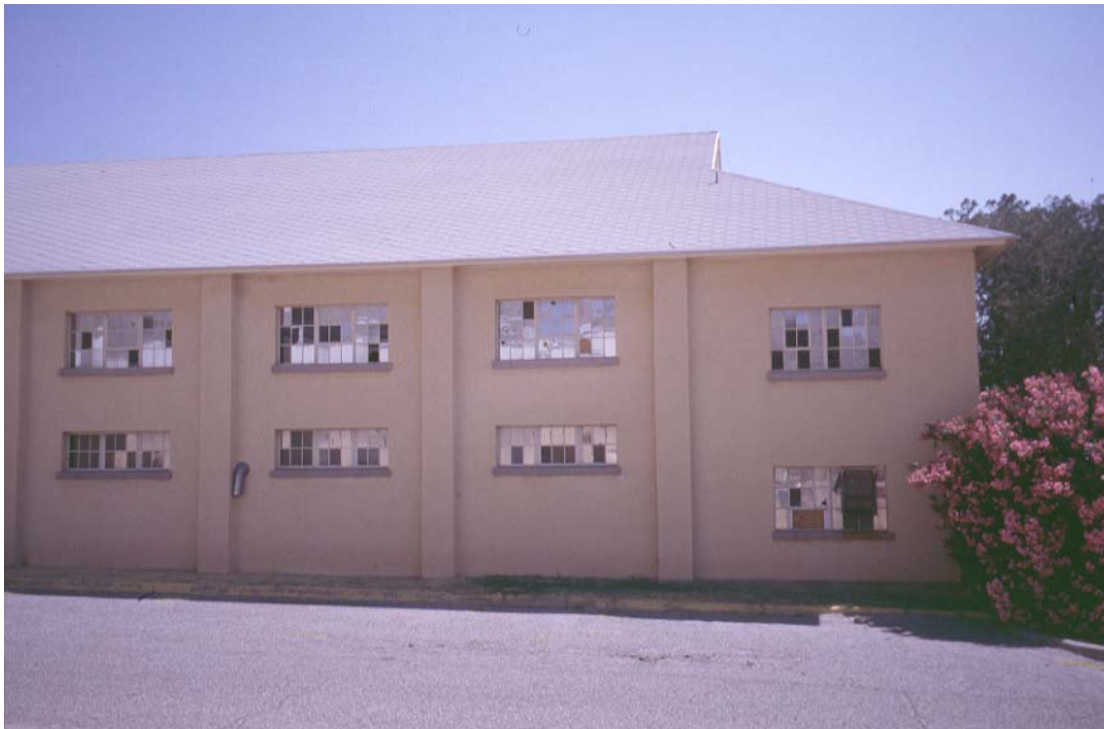
Photograph 25. Inconsistent use of film on gymnasium windows.
