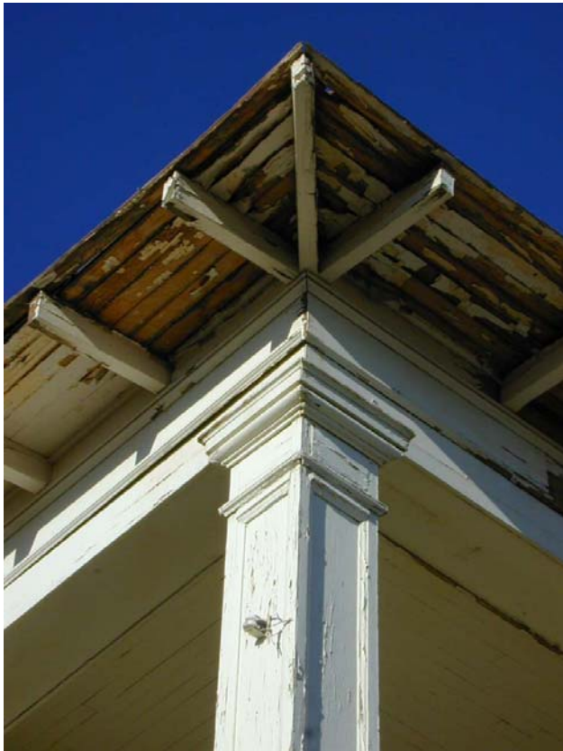
Photograph 46. Typical barracks porch roof damage.
