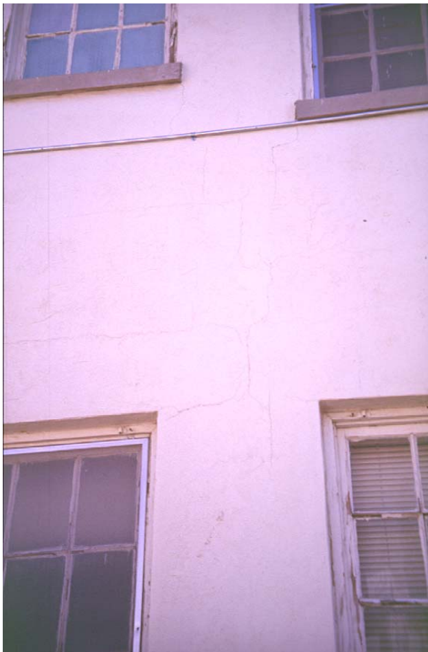
Photograph 39. Typical minor stucco damage on barracks exterior.
