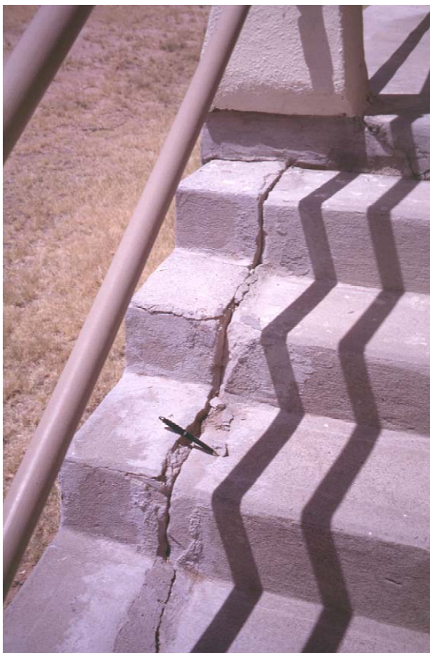
Photograph 74. Badly cracked Conference Center stairs.
