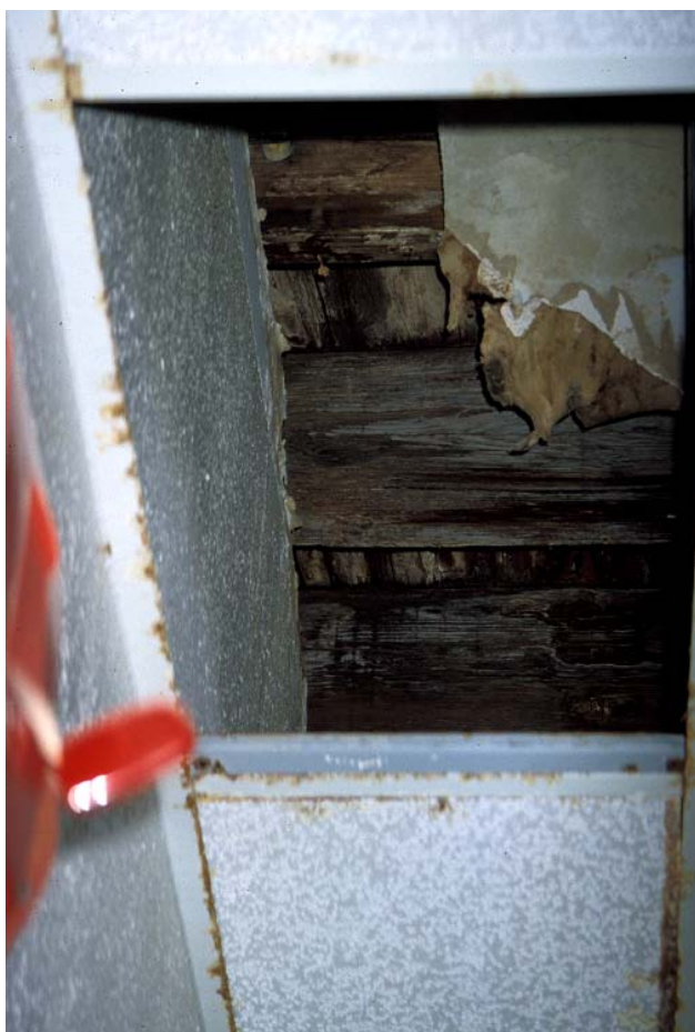
Photograph 45. Typical water-damaged barracks ceiling in first-floor washroom.
