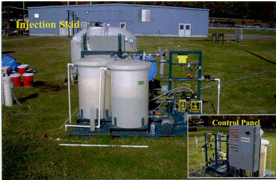
Figure 16. Control Panel and Treatment Skid
