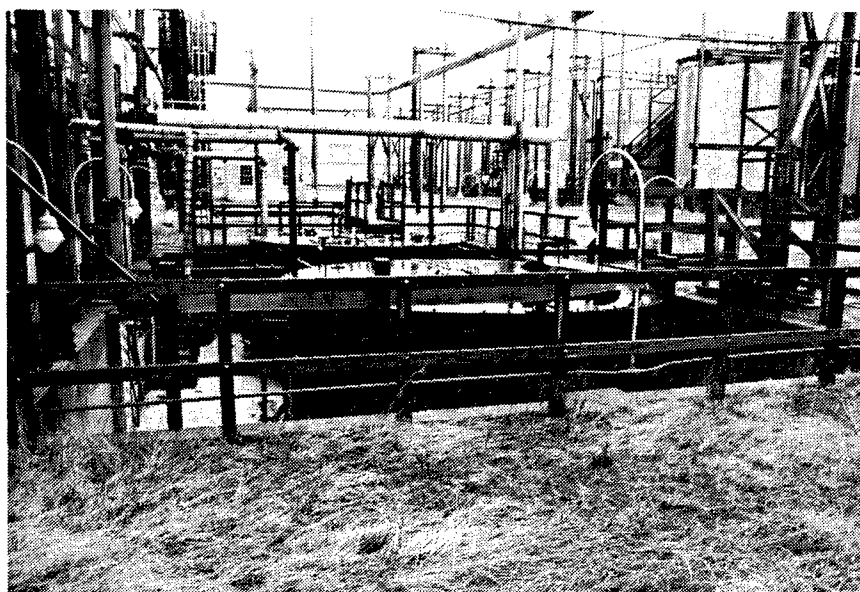
Figure 28. Building 704-1: Cooling product tank for 92% sulfuric acid.
