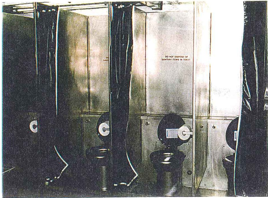
Figure C-2. Low Water Flush Toilets
