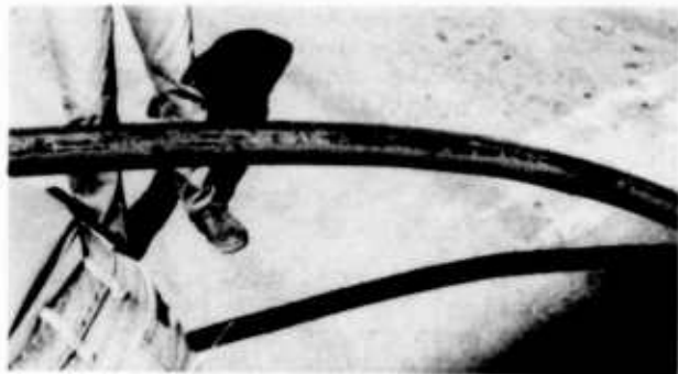
FIG. 4 BONDED ASP EMERGING FROM CABLE DUCT
