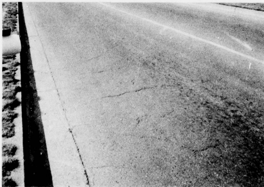
Photo 30. Fort Lewis--type cracking in pavement surface on Second Division Drive
