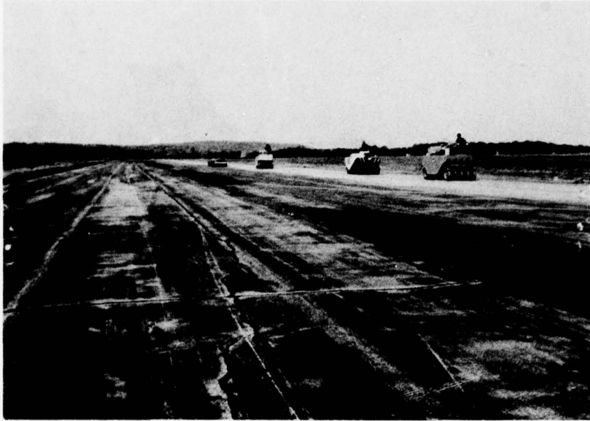
Photo 17. Fort Devens--rolling of chips and sweeping of joint prior to application of next lane
