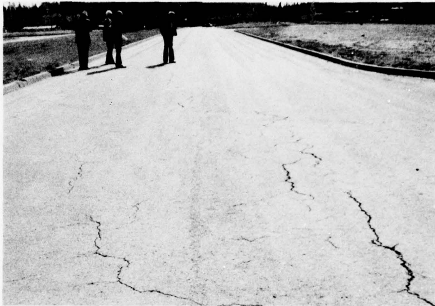
Photo 31. Fort Lewis--cracking in pavements on Faith Avenue; most of cracks in localized areas
