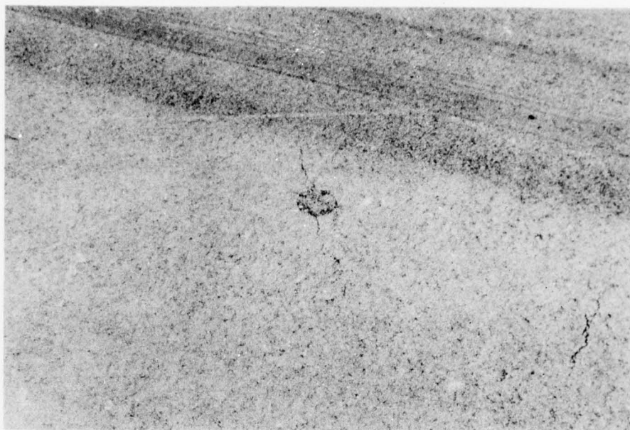
Photo 61. Fort Lewis--fine hairline crack created in overlay by wrinkle in Mirafi 140 fabric
