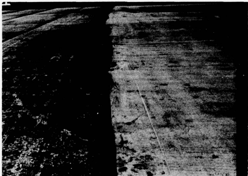
Photo 11. Fort Devens--joints and splices in fabric sections sealed with joint seal material to glue edges to pavement
