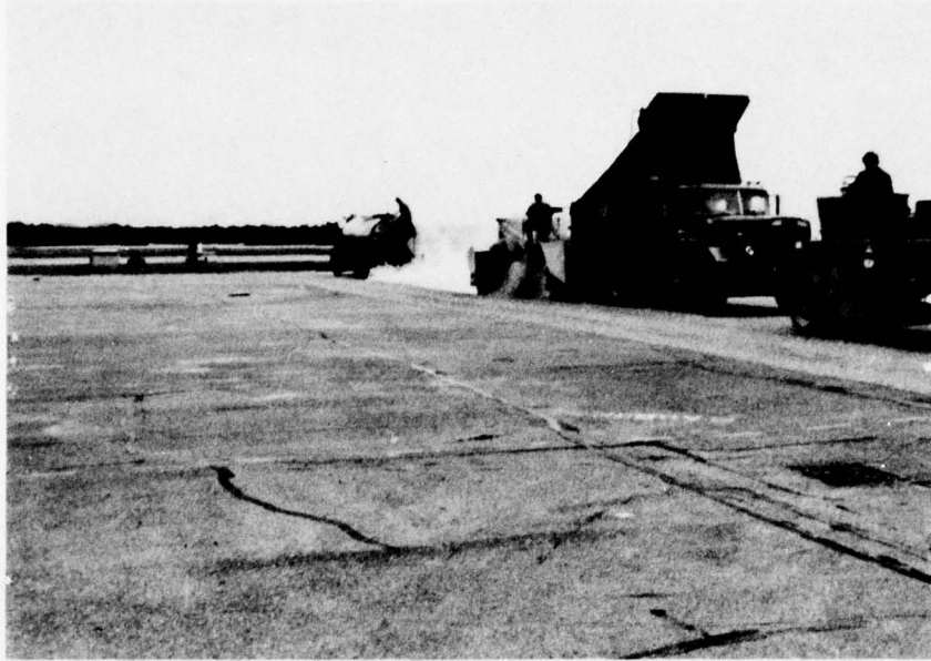
Photo 19. Fort Devens--placement of asphalt rubber and chips, and rolling of U. S. Rubber test area on apron
