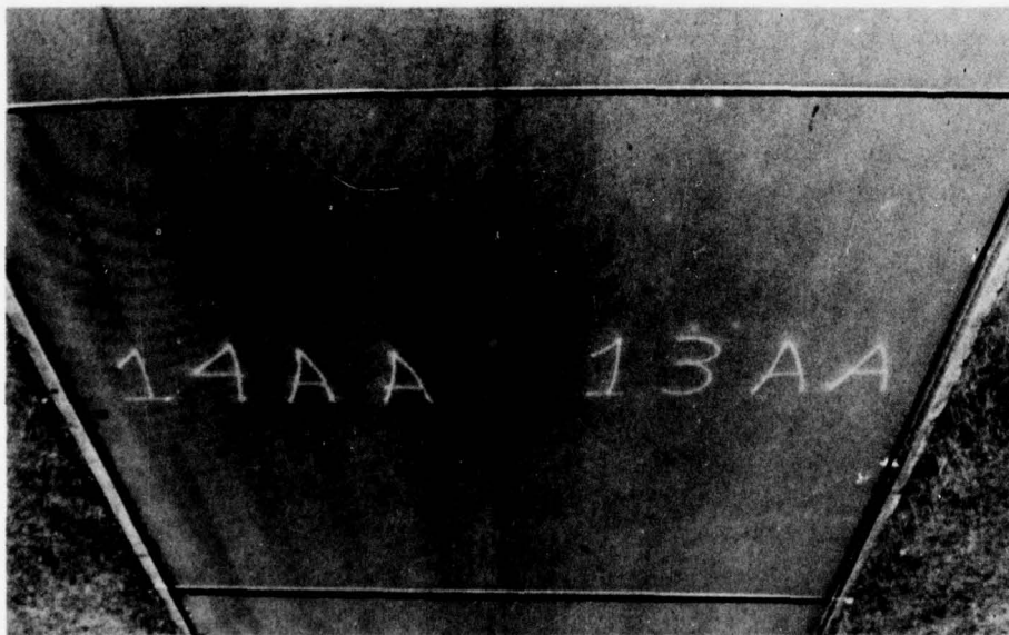
b. Condition of surface 6 months after overlay
