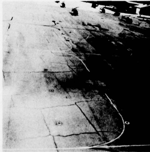
Photo 20. Fort Stewart--crack pattern from soil-cement base
