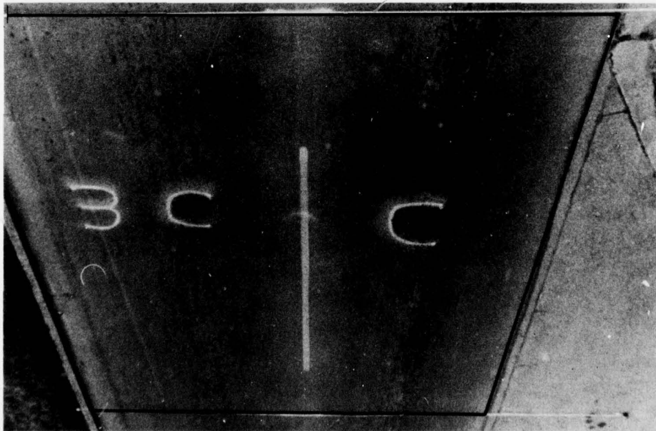
b. Condition of surface 6 months after overlay
