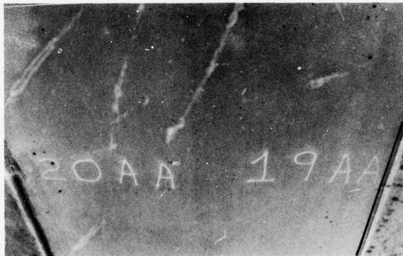
b. Condition of surface 6 months after overlay
