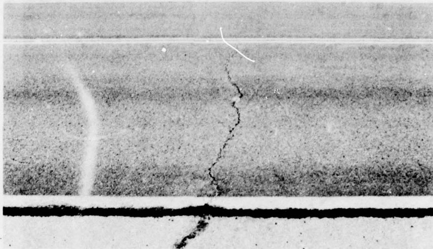
Photo 116. Fort Devens--reflected crack in Barnum Road outside of test areas
