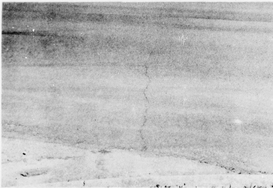
Photo 63. Fort Lewis--reflection crack in control section on north side of Faith Avenue
