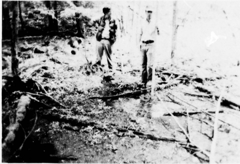
E. Seepage at Toe of Dam
