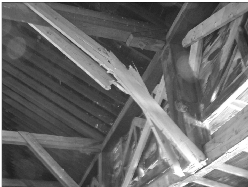
Figure 5: Structurally Unsound Warehouse at Fort Leavenworth, Kansas
