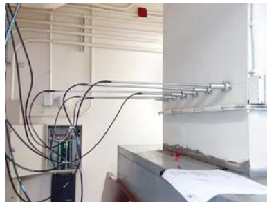
(c) Installed brackets with holding velocity probes
