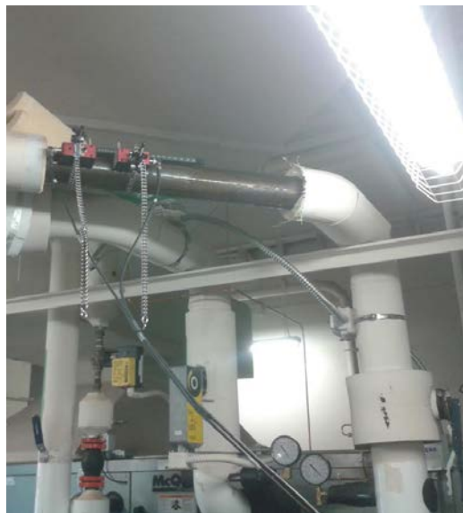
Installed ultrasonic meter
