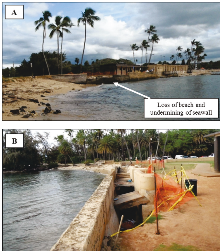
Figure 3. Pictures from the March 2017 site visit showing the severe erosion of the beach at the northern section of the Haleiwa Beach Project (A) and the washed out area behind the seawall (B).
