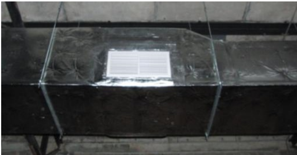
Figure 5. Ducting vent showing left-to-right size transition from larger to smaller.
