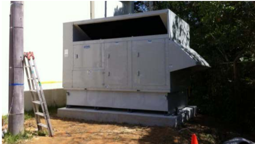
Figure 2. Selected dehumidification unit on concrete pad.
