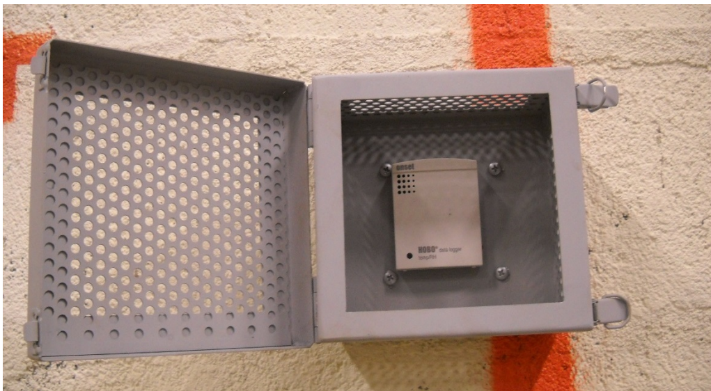
Figure 8. Interior temperature and humidity sensor mounted in protective box.
