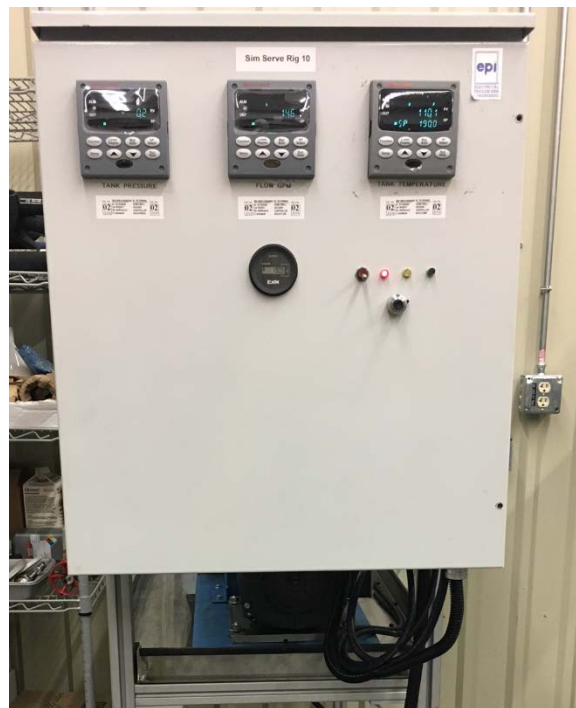
Figure 4. Front of Rig Showing Instrument Panel
