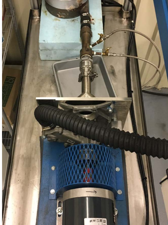
Figure 3. Pump Connection to Calibrated Flow Meter
