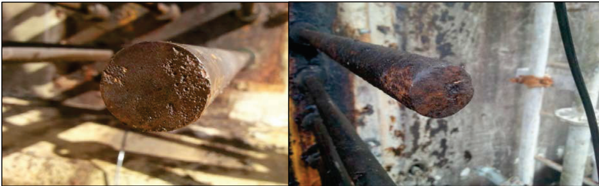
Figure 4. Pitted rod and surface corrosion on rod.
