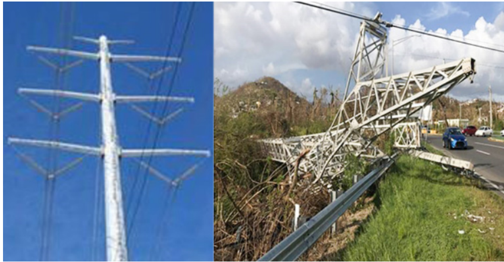
Figure 9. Collapsed Transmission Tower in Puerto Rico 101
