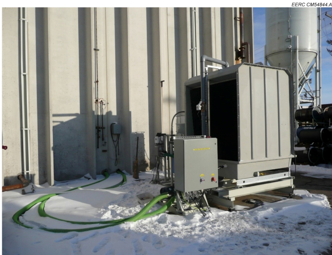
Figure 10. Tower and pump skid with electrical cabinet.
