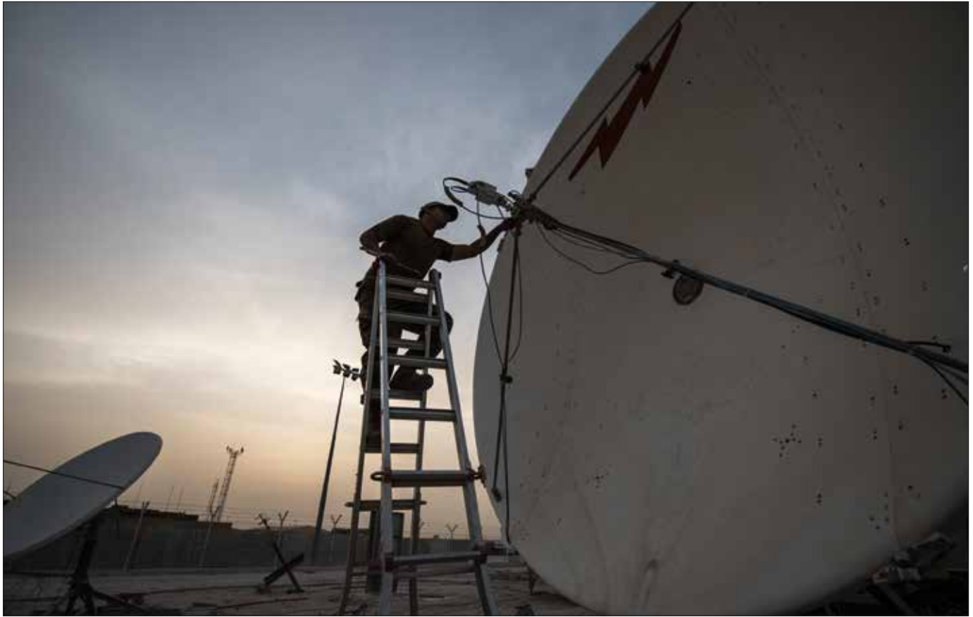
Airman with 379 th Operations Support Squadron performs maintenance on satellite dish at Al Udeid Air Base, Qatar, March 30, 2018, as part of Operation Silent Sentry , protecting critical satellite communication links (U.S. Air National Guard/Phil Speck)
