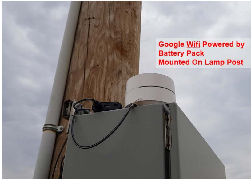
Figure 66. Placement of Google WiFi Mesh Router above the Electrical Distribution Board Mounted on the Lamp Post between the Two-Level Building and the Training Shed
