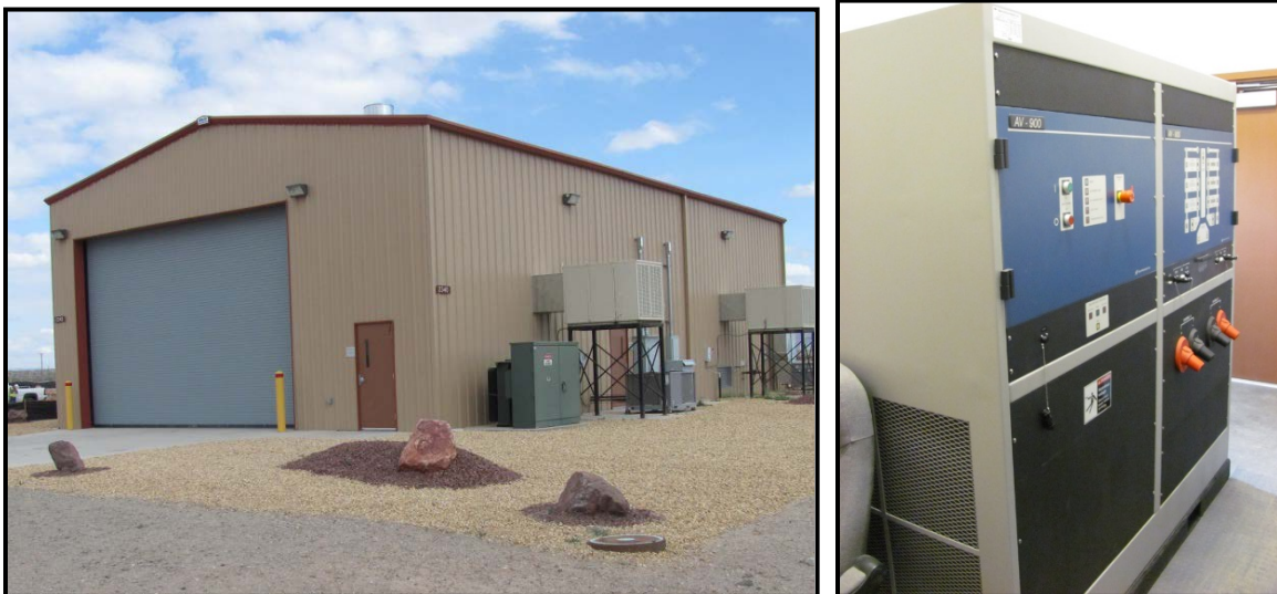
Figure 189. Hybrid Electric Facility (left) and AV900 Load Bank (right).
