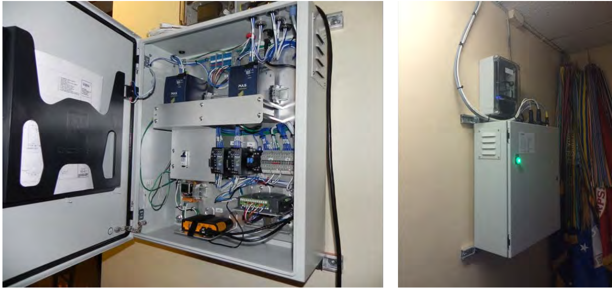
Figure 19. Control Panel (with Power Supply and Network Controller) Installed
