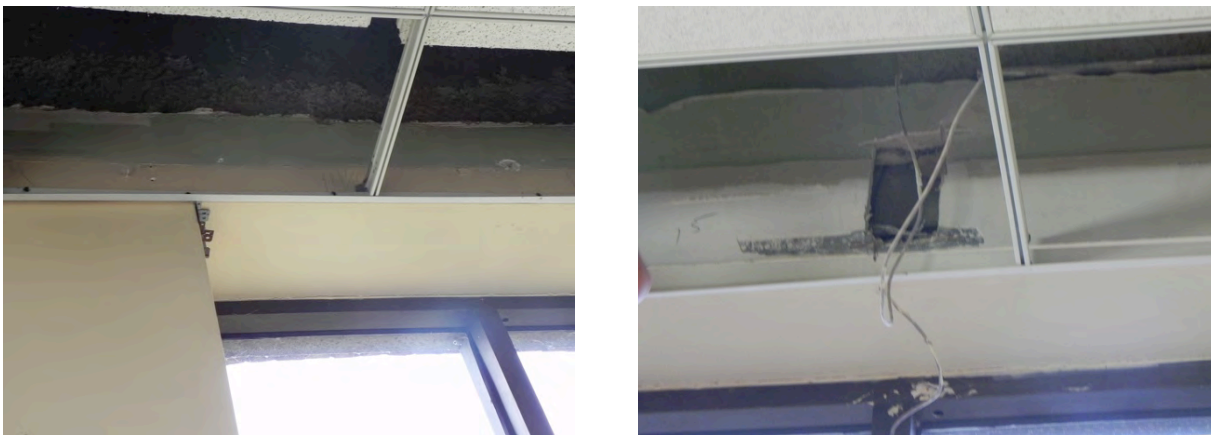
Figure 16. Available Space for Dynamic Glass System Components in the Existing Ceiling Plenum
