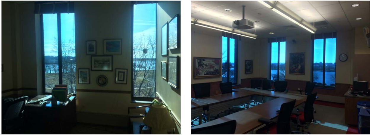
Figure 25. Glass Appearance as Commissioned – Fully Tinted
