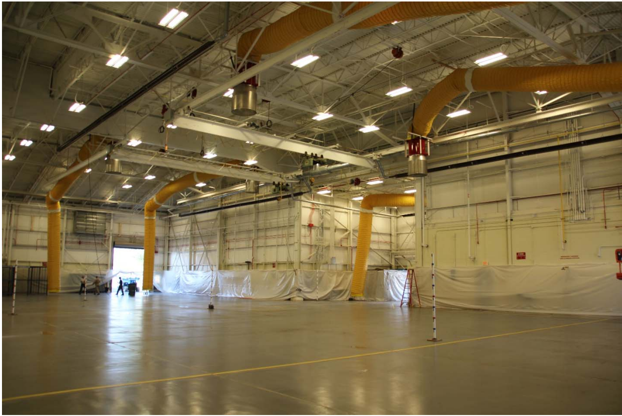
Figure 3. Protective Curtain on Hangar Boundaries
