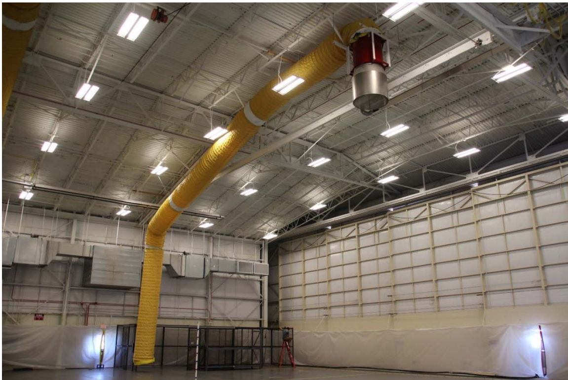
Figure 10. Typical Ductwork Arrangement
