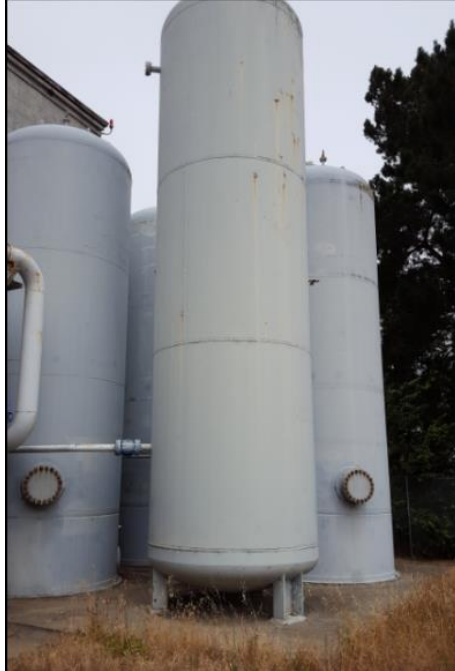
Figure 35. Air Storage Tanks.
