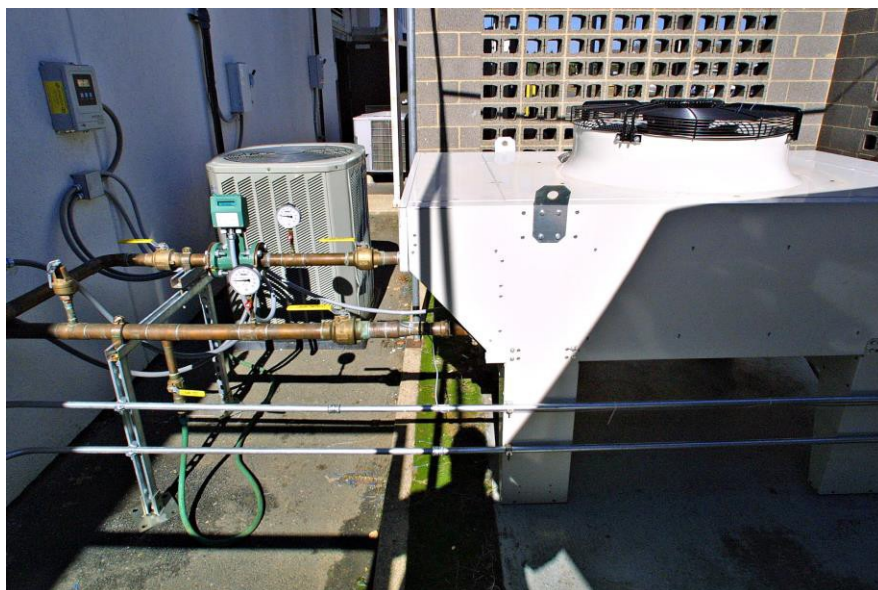
Figure 4-3: Dry Cooler Outside of NRL Data Center
