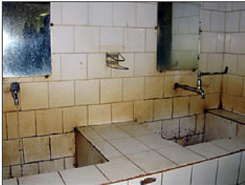
Figure C27. Inadequate and unequipped sinks at Chittagong Medical Hospital, Bangladesh, before implementation of the WHO hand hygiene improvement strategy (www.who.int, 2016).
