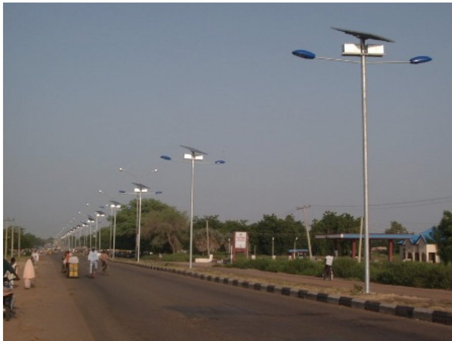
Figure C2. Solar-panel street lights in Nigeria (prlog.org, 2008).
