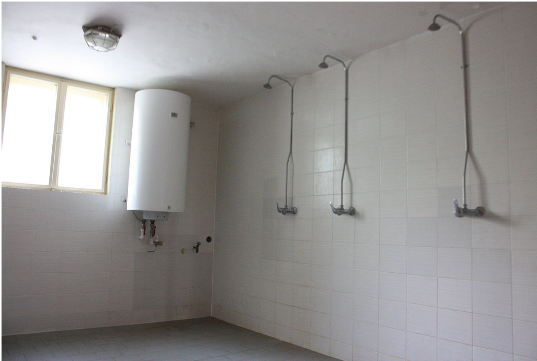
Figure C28. Communal shower at Gymnazium Brno-Řečkovice, Czech Republic (commons.wikimedia.org, 2009).
