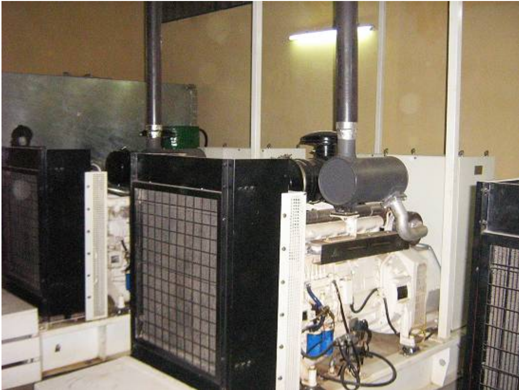
Figure C3. Communal biofuel generators in Garalo, Mali (homepower.com, 2010).
