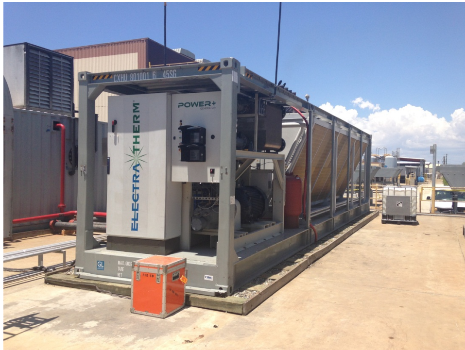
Figure 6. ORC Unit Installed at GTMO
