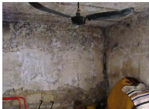
Figure 2-8. Burned interior of Jassim’s brother’s house 41
