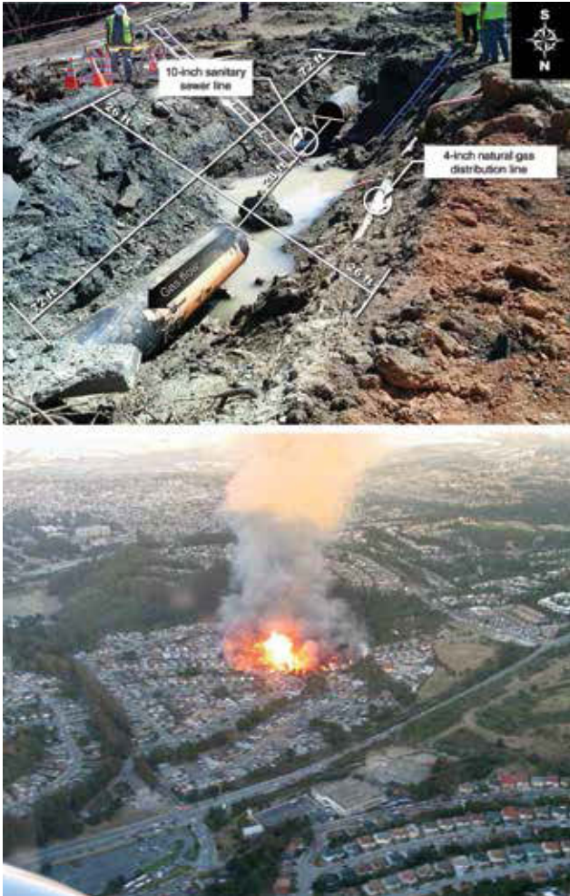
Figure 6. PG&E gas transmission pipeline explosion. Crater and ruptured pipeline ( top ) and aerial view of fire ( bottom ). (Reproduced from National Transportation Safety Board [NTSB], Pacific Gas and Electric Company Natural Gas Transmission Pipeline Rupture and Fire, San Bruno, California, September 9, 2010 , Pipeline Accident Report NTSB/PAR-11/01 [Washington, DC: NTSB, 30 August 2011], 1–2, http://www.nts.gov/investigations/AccidentReports/Reports/PAR1101.pdf .)
