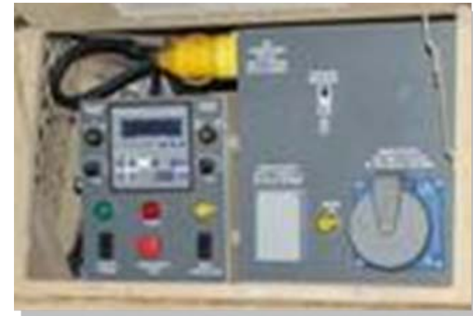
Interface and Control Panel
