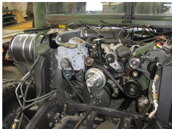
Alternator + belt driven HV generator
