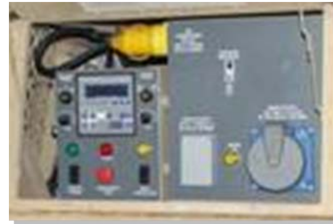
Interface and Control Panel
