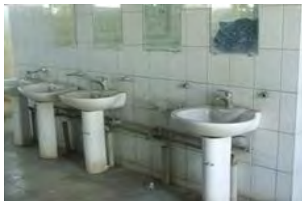
Photo 2 - Poorly Maintained Facilities in Bathroom Building 7
