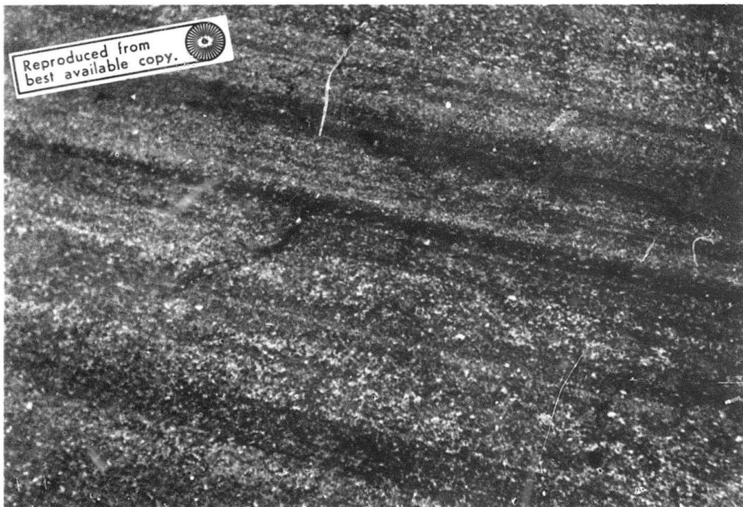
Photograph 3. Distressed area near north end of runway
