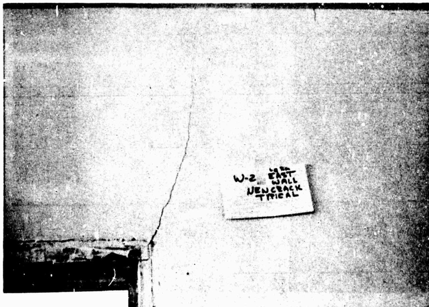
Fig. 20 W-2, Typical new crack
