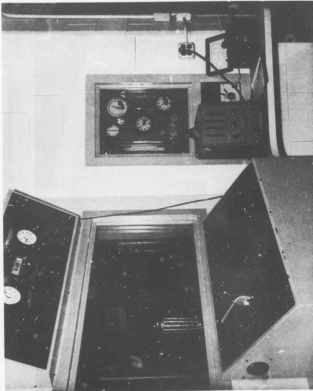
Figure 12. Laboratory Control Room and Pump Instrumentation.
