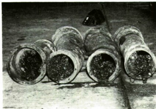
FIG. 5. Seawater pipes partially blocked with mussel fouling
