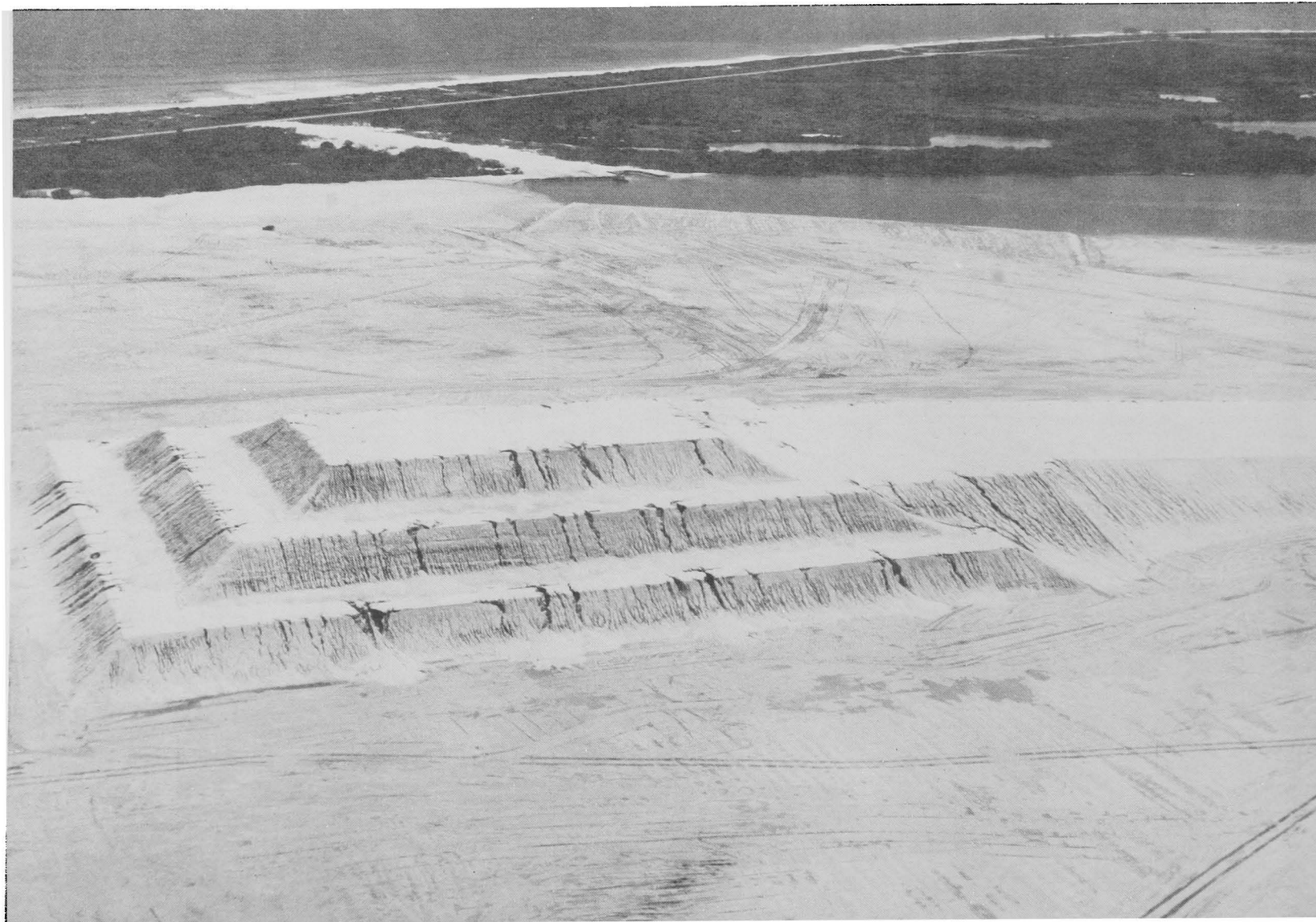
Reminiscent of an ancient pyramid, this accumulation of 500,000 cubic yards of surcharge fill occupies the site of 39-A. Dredged from Banana River, the surcharge pile placed a 1.5 billion pound load on the construction site. When the pyramid had settled the pad area about 4 feet, the surcharge was removed and construction began.
