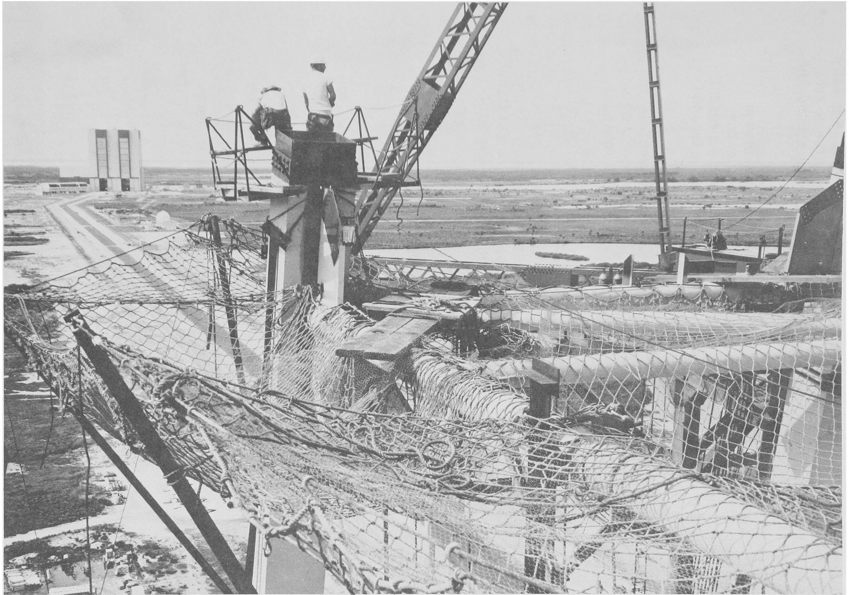
Feature of Mobile Service Structure construction was safety net to halt the fall of steel sections or personnel during construction. It was built in the "park" position south of Crawlerway and about a mile from Pad 39-A.
