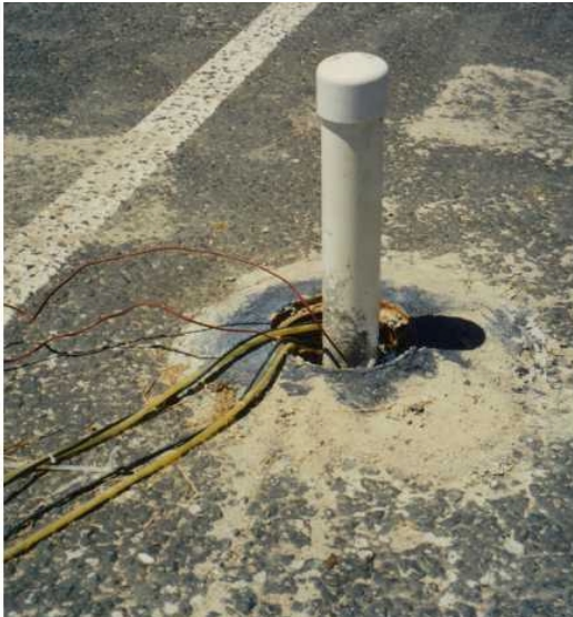
Photo 9. Oxygen sensor/VMP surface completion.
