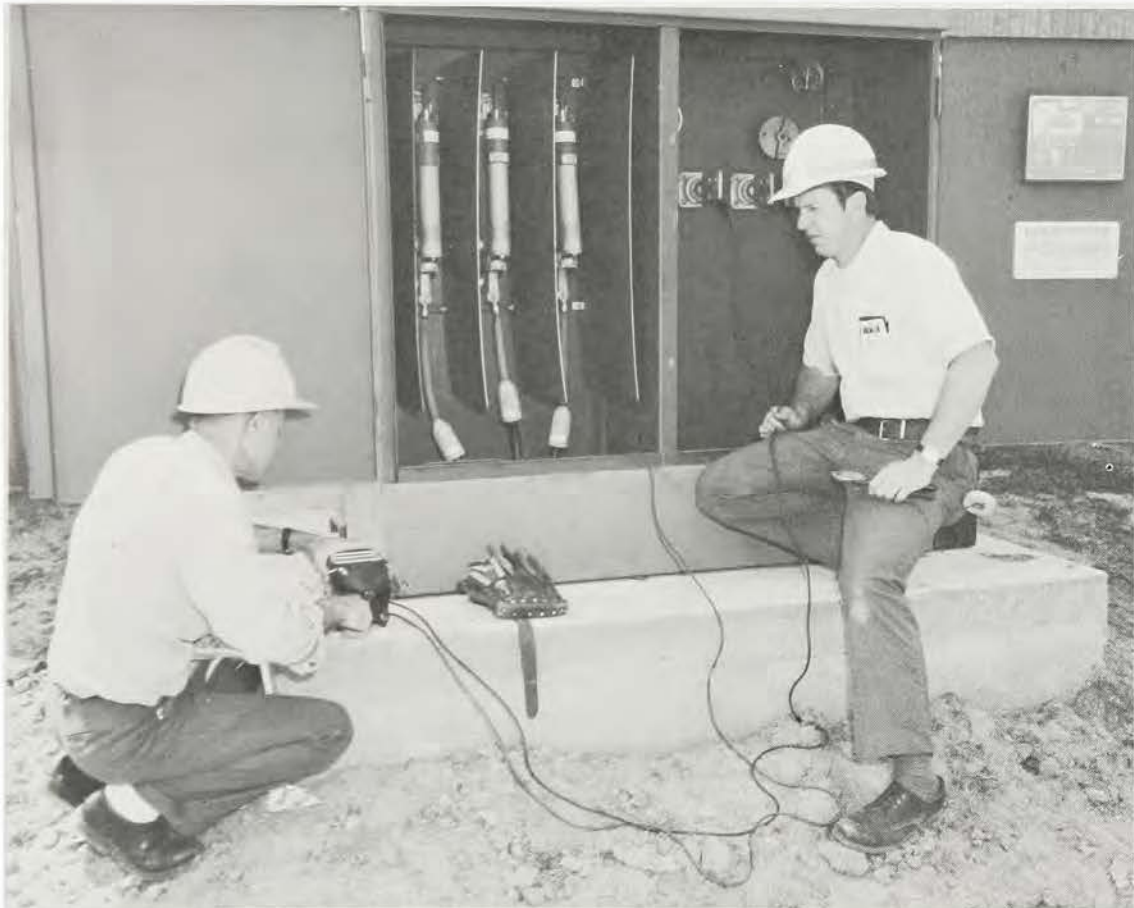
Engineering and Construction Services Division electricians check the insulation value of wiring in the power substation for WES' new Advanced Scientific Computer
