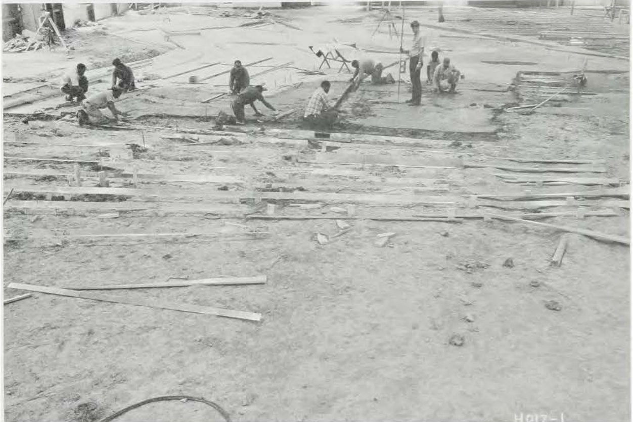
Construction of McAlpine Locks & Dam Model, Ohio River. Skilled model makers use metal templates cut to the proper scaled elevation to duplicate nature. Concrete is placed between the templates and molded to their contours to form the model surface
