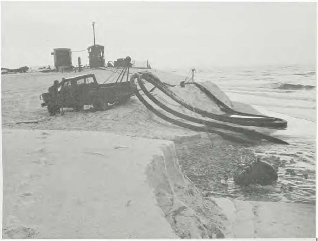
Sand bypassing system
